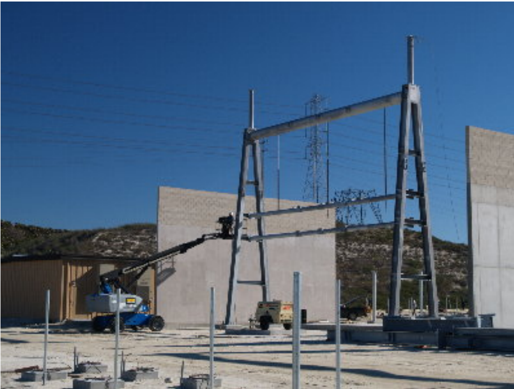
Figure 2 – The large racks have been raised and a crew worked to prepare the racks for cable.
