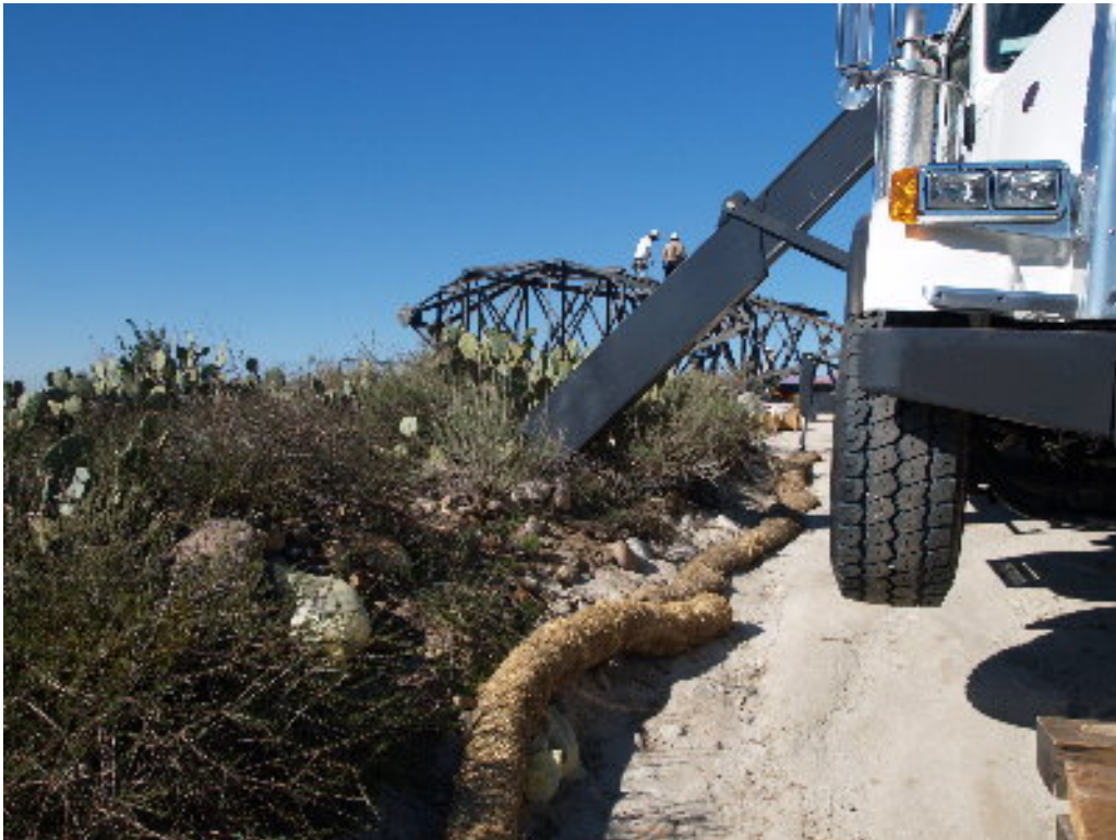
Figure 8 – A mobile crane outrigger was set off the access road into the vegetation on the 220 kV transmission corridor.
