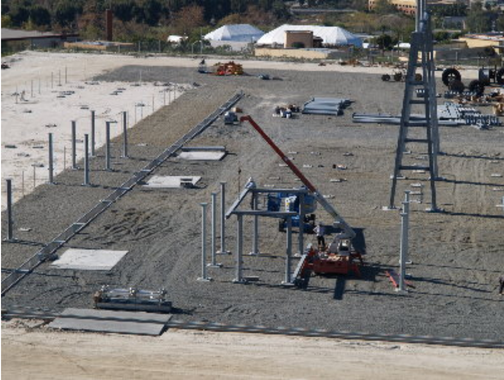
Figure 1 – A small crew worked with a crane to set the horizontal sections on the supports on the southern end of the substation site.
