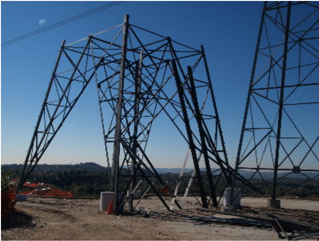
Figure 7 – The upper section of the middle lattice structure on the 220 kV transmission corridor has been assembled and is ready to raise.
