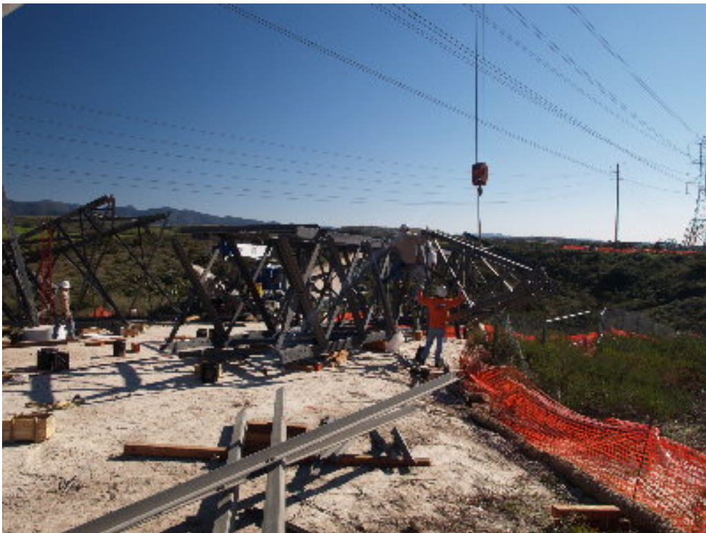
Figure 6 – Crews worked on the ground to assemble the upper section of the northern lattice structure on the 220 kV transmission corridor.
