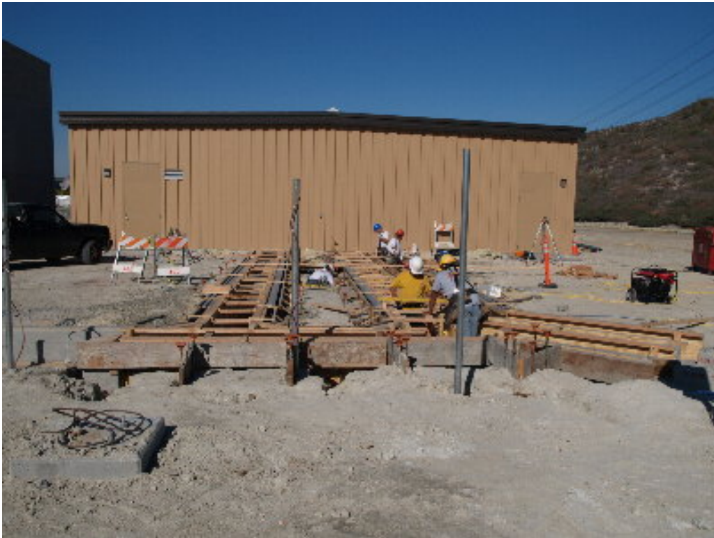
Figure 3 – A larger crew worked to rebuild the trench forms leading into MEER #1.
