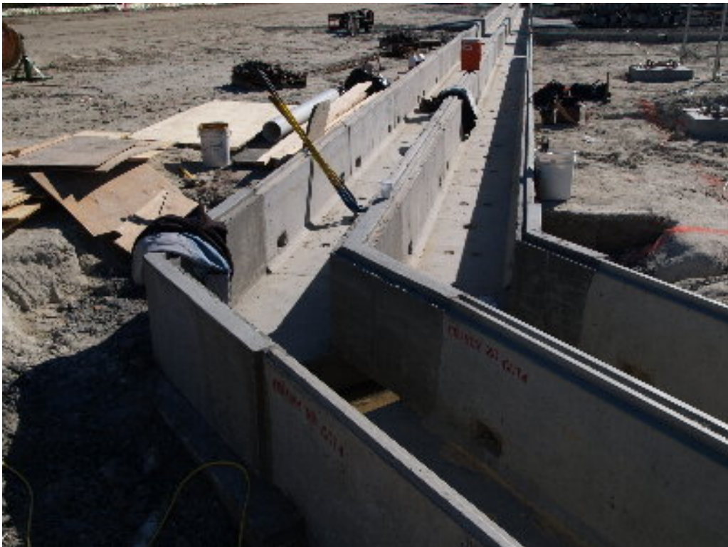
Figure 4 – The pre-cast concrete sections of trench need to be connected by formed sections at angles and intersections (see darker formed angle).
