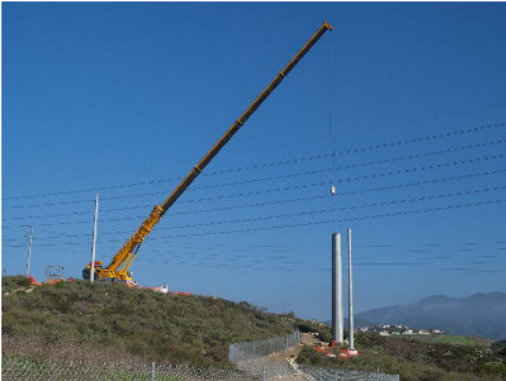
Figure 4 – Hill Crane set the steel pole sections on the foundations southeast of the substation site.
