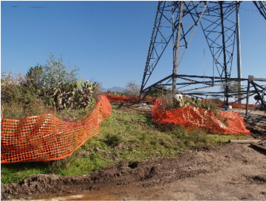
Figure 7 – The proposed crane access at the lower lattice structure on the 220 kV transmission corridor has been delineated.
