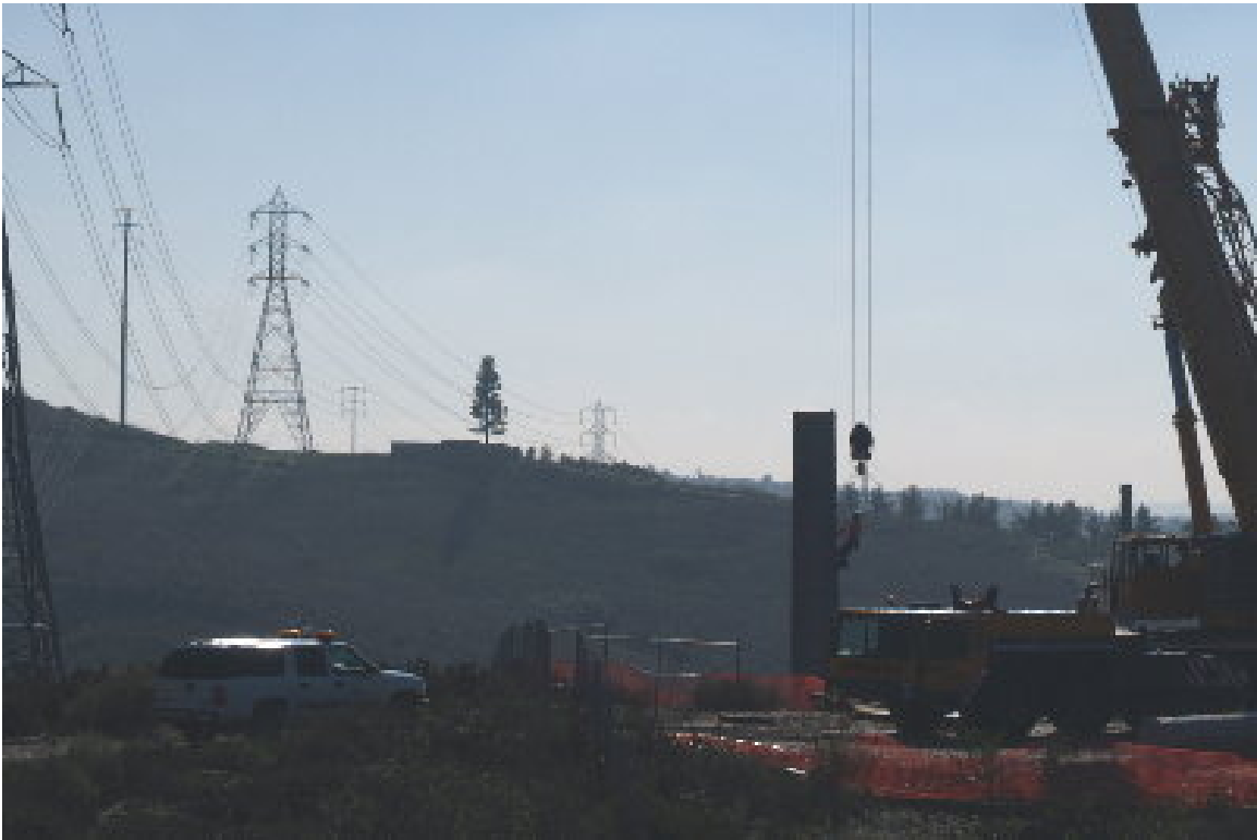
Figure 5 – Workers prepared the steel towers for the upper sections once the lower sections were secured.
