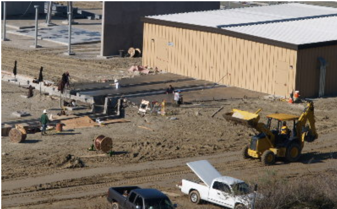
Figure 2 – A larger crew worked on finishing the concrete slab outside the south wall of MEER #1. The backhoe operator worked on maintaining the access road.
