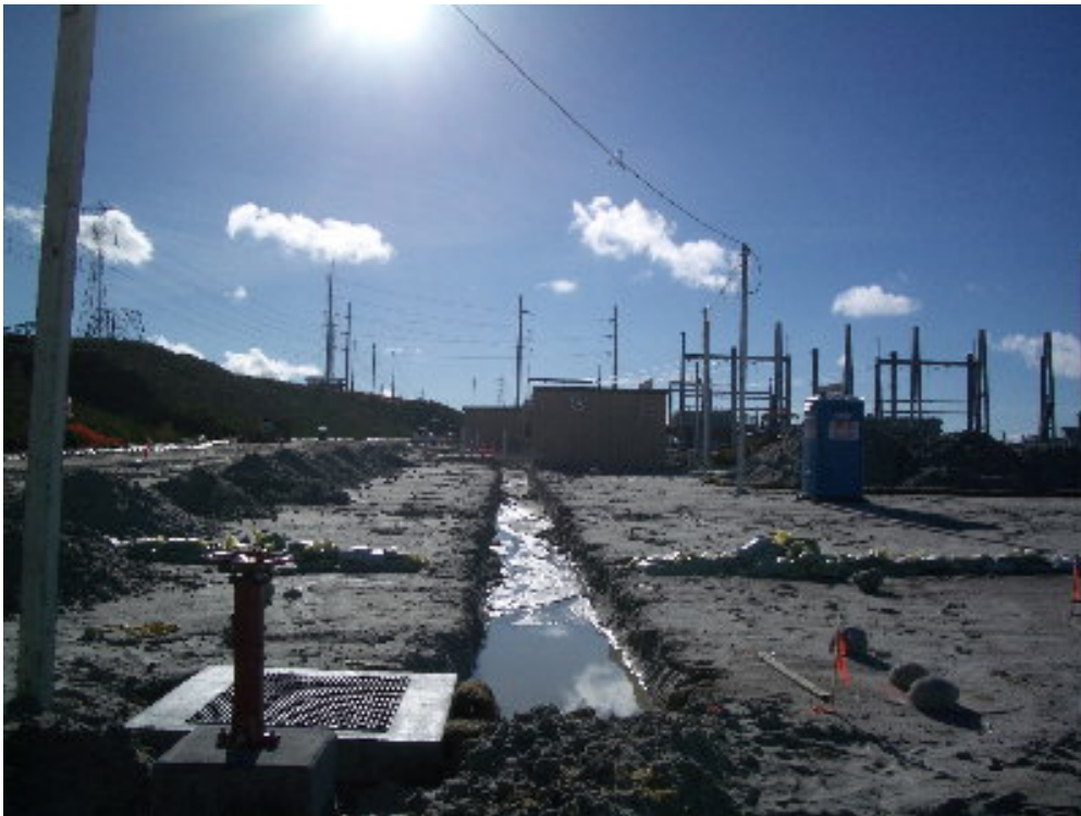
Figure 2 – Recently excavated trenches have filled with storm water.
