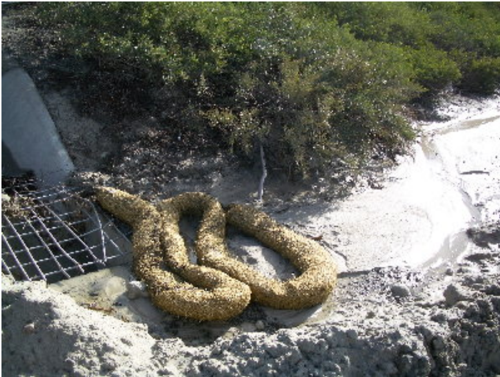
Figure 3 – Loose spoils had been placed to direct water into the storm drain without proper sediment control devices in place.
