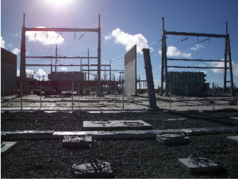
Figure 1 – Crews set the first A transformer onto the pad prior to the rain.
