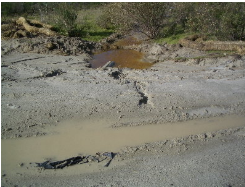
Figure 4 – BMPs are required at the culvert crossing near the substation back gate.
