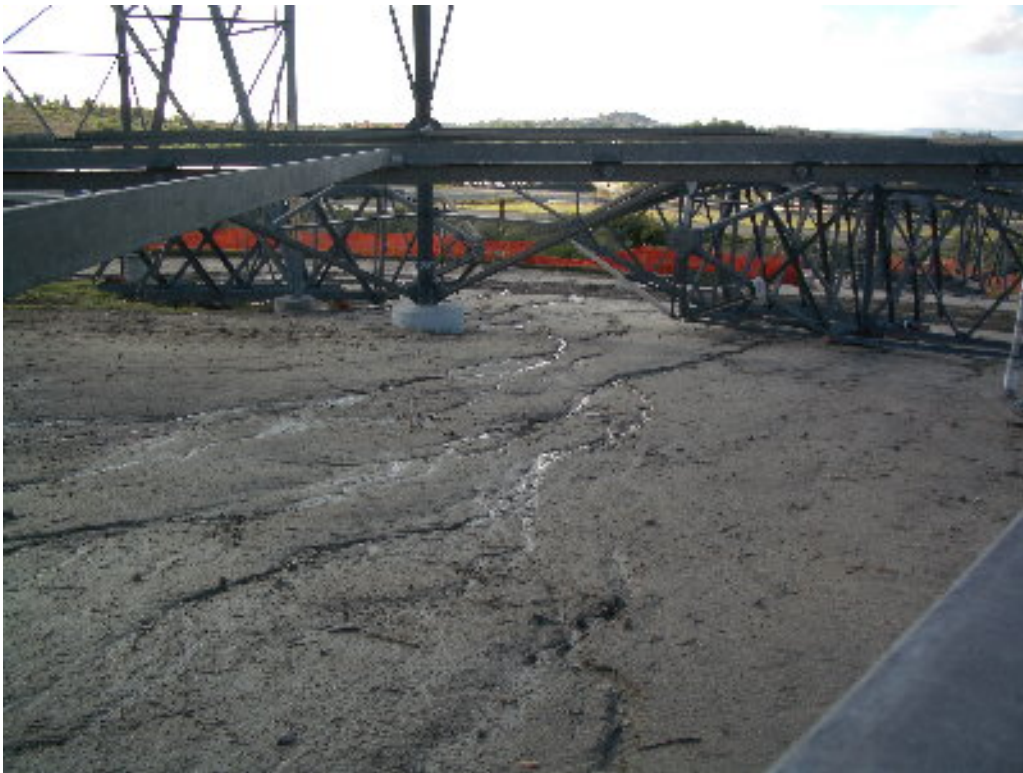
Figure 6 – Minor erosion from the lattice tower pad flowing into the recent vehicle ruts.
