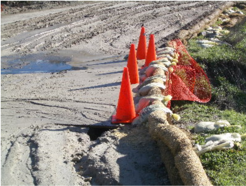
Figure 5 – Erosion from 220 kV access road has bypassed BMPs and sediment has entered the drainage.
