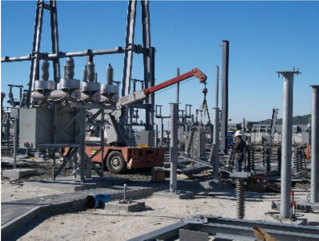
Figure 1 – A small NRG crew worked with lifts to prepare the 220 kV circuits.
