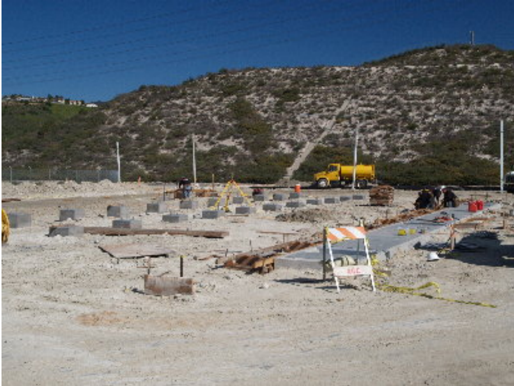
Figure 3 – Kindness worked on the 12 kV foundations on the northern section of the substation site.
