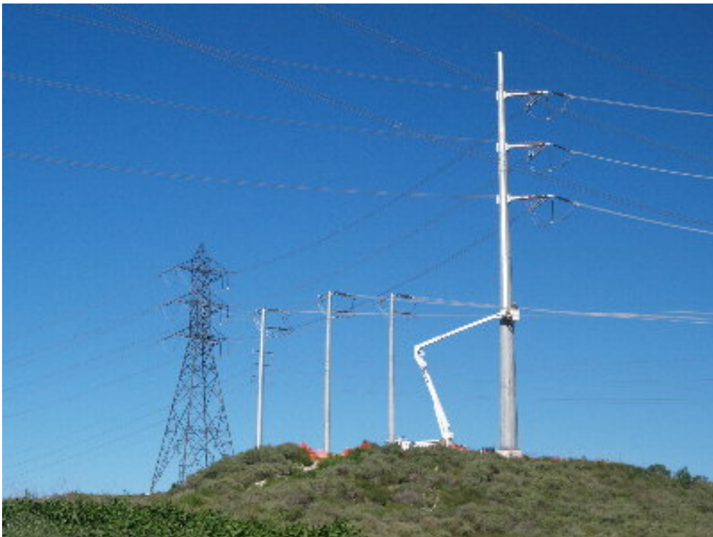
Figure 4 – The transmission line crew worked in a man-lift to on the large turning pole.
