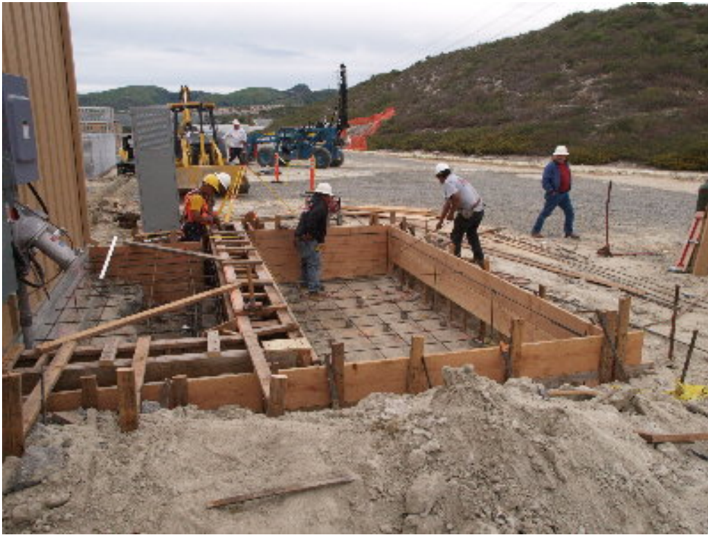
Figure 3 – Kindness worked on the cable trench entering MEER #1. The trench will replace the conduit that was too small for the number of cables entering MEER #1.
