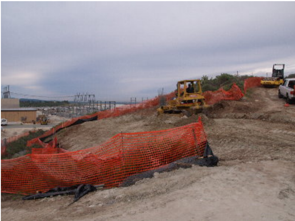
Figure 6 – A small bulldozer was used to cut the pad for the 66 kV pole.
