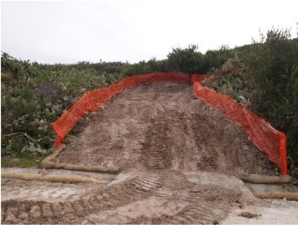
Figure 7 – The BMPs originally installed on the 66 kV right-of-way will need improvement to handle the predicted rain events.
