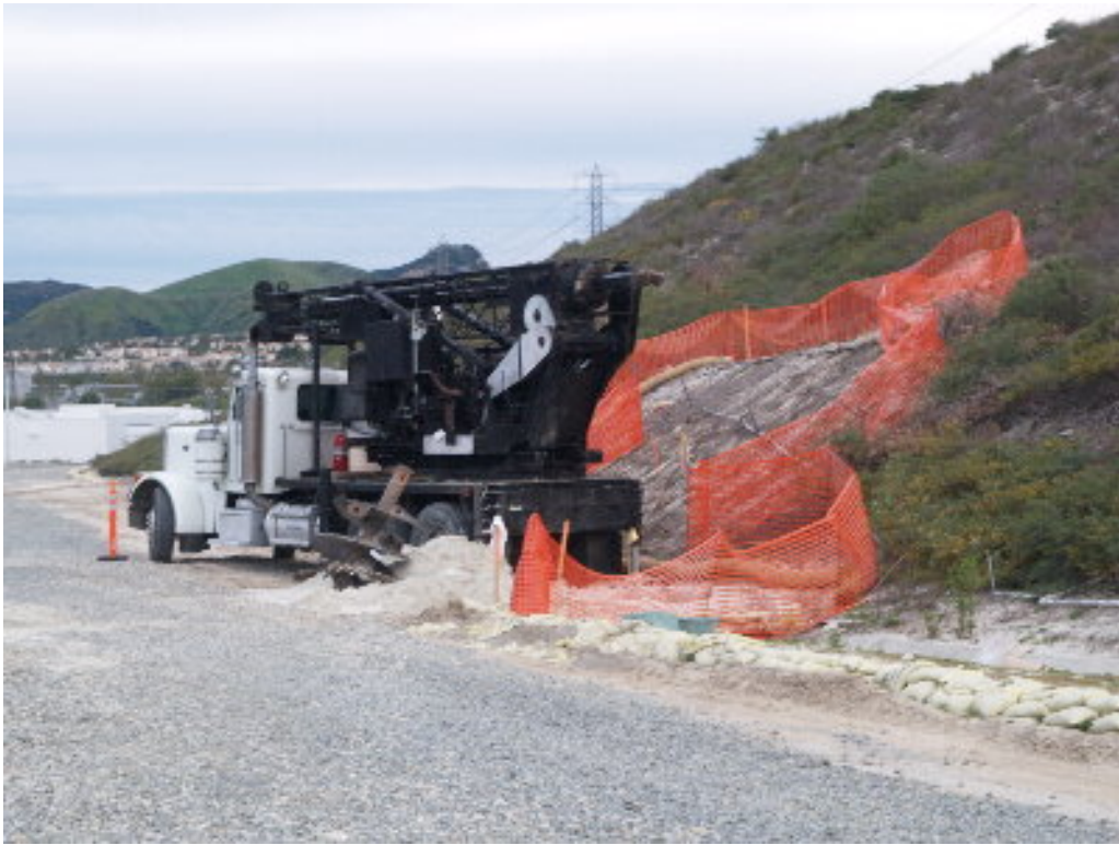
Figure 5 – The drilling contractor worked to excavate the foundation for the 66 kV poles.
