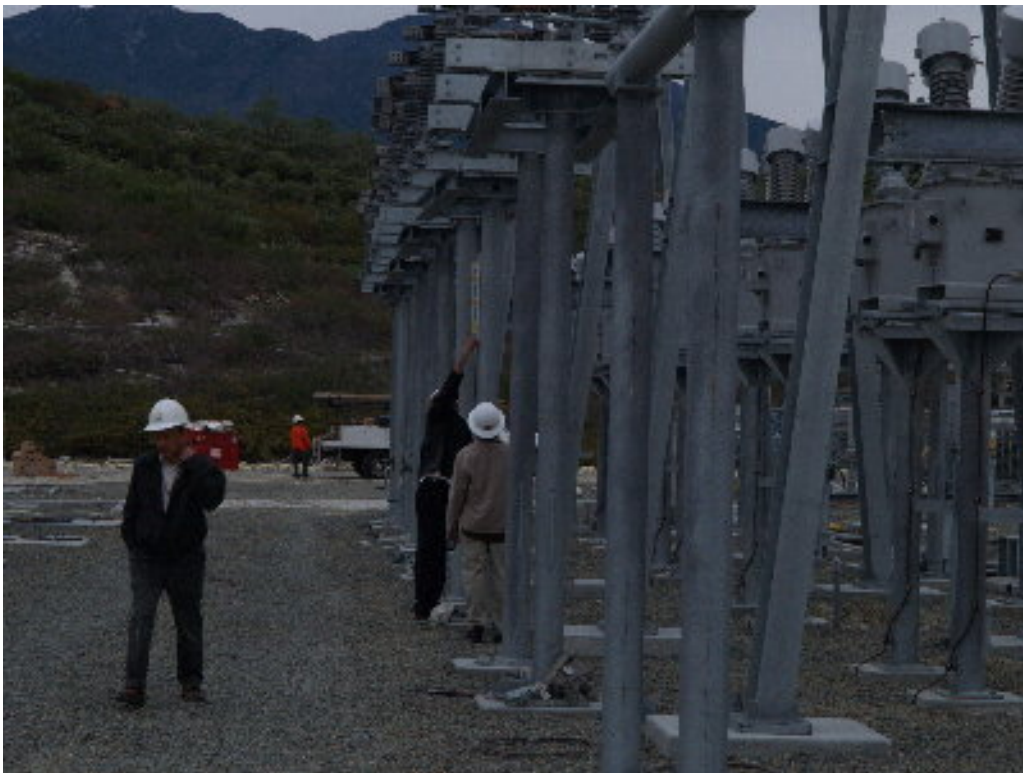
Figure 4 – Engineers reviewed the poles that were out of plumb due to fabrication errors.
