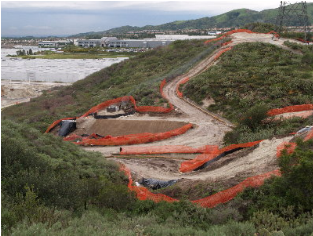
Figure 5 – Pads have been graded and one foundation poured on the 66 kV transmission line corridor.
