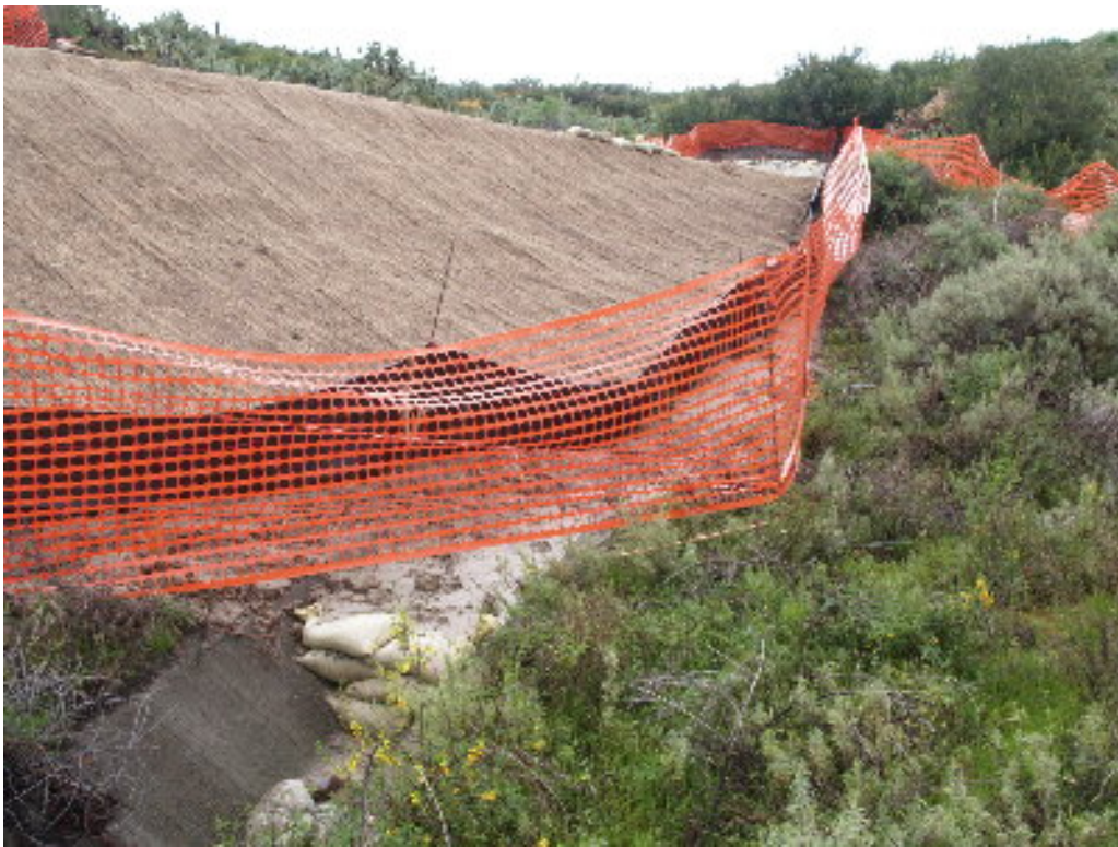
Figure 6 – The BMPs originally installed on the 66 kV right-of-way will need improvement to handle the predicted rain events.
