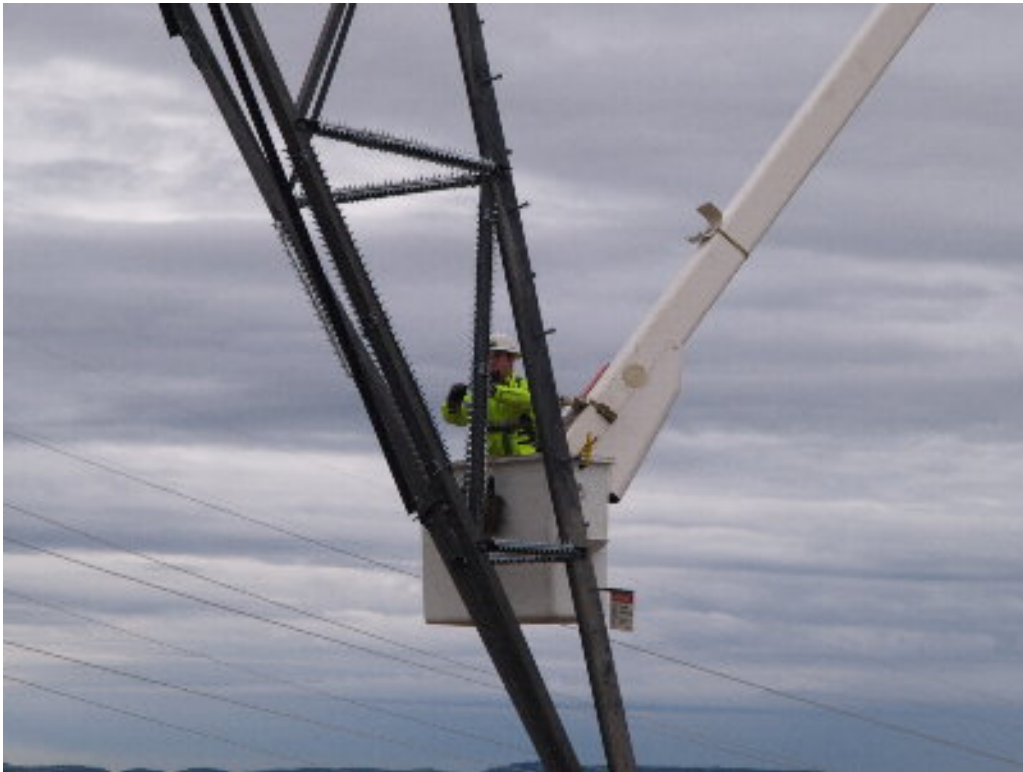
Figure 3 – The 220 kV construction contractor worked to install climbing deterrents on the lattice towers.
