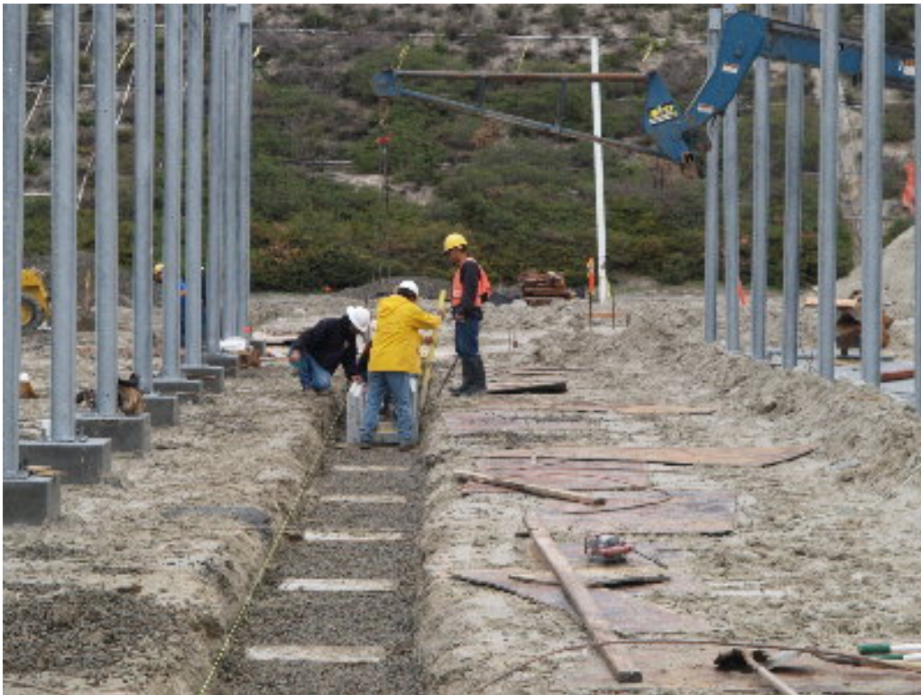
Figure 2 – The Kindness crew worked to place and adjust the pre-formed concrete trenches for the 12 kV section of the substation.
