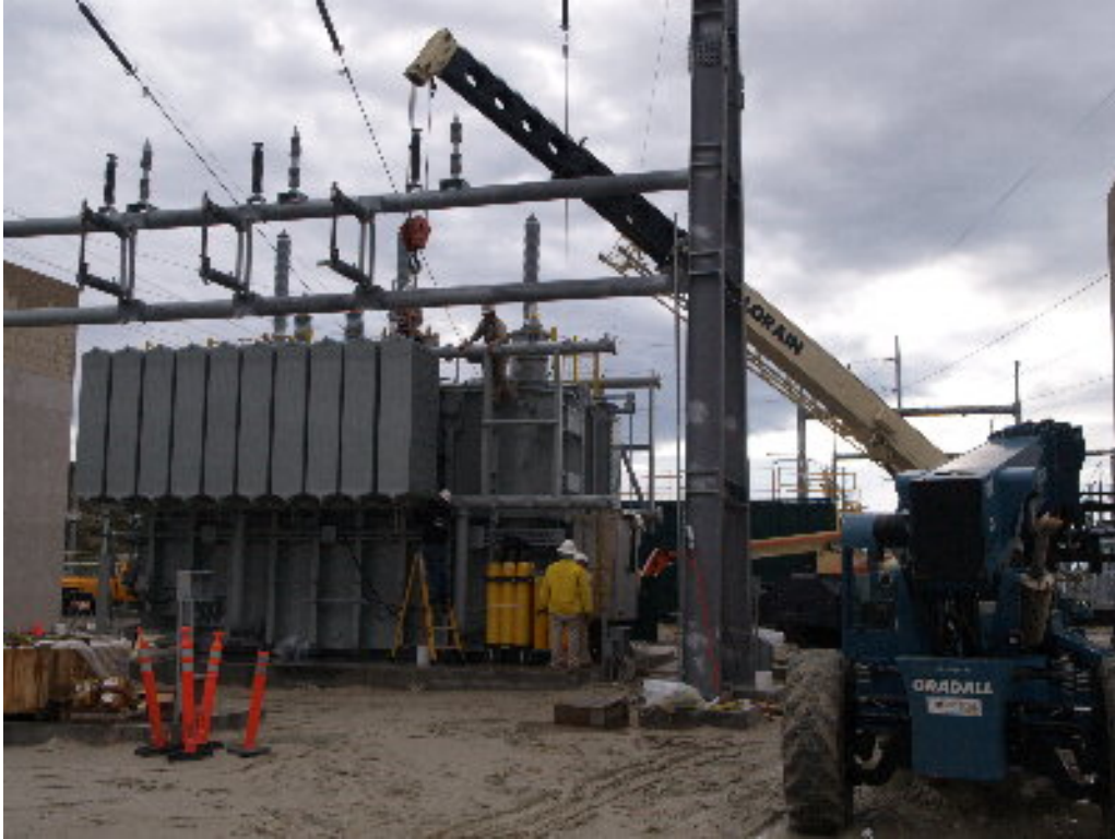
Figure 1 – A SCE crew worked to install the external cooling fins on the A-bank transformers.
