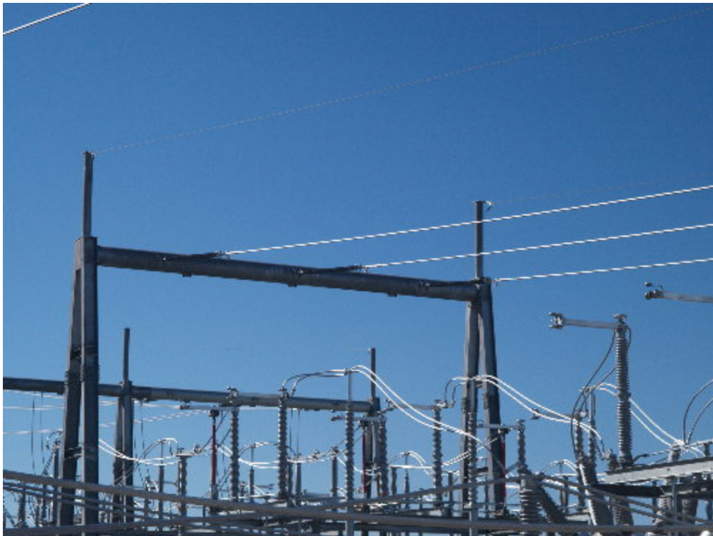
Figure 4 – The circuits on the risers connecting the 220 kV portion to the rest of the substation site have been removed for safety.
