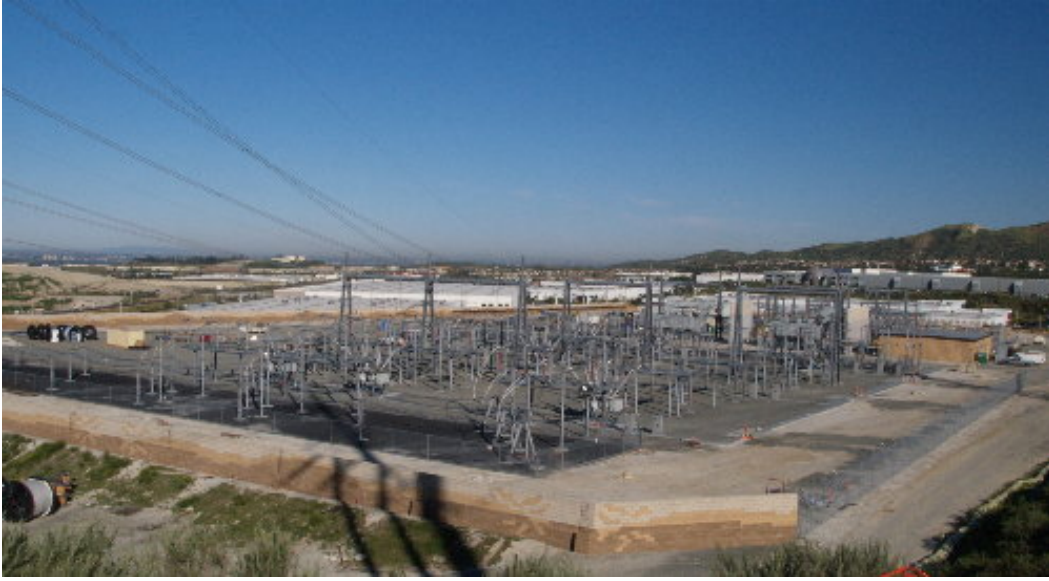
Figure 1 – Overview of the substation site as of April 1, 2005. Only limited work was occurring on the substation site during the site visit.
