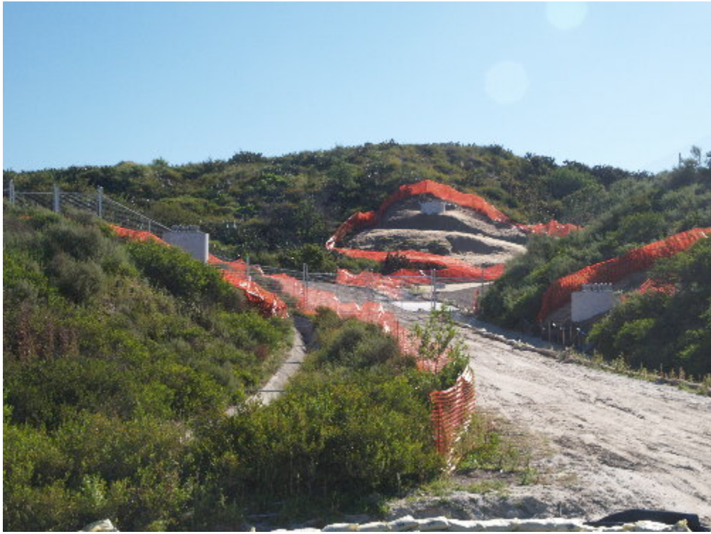
Figure 5 – The cyclone fence on the hillside above the substation site was replaced.
