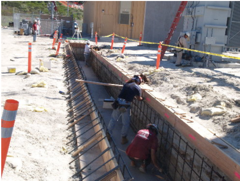
Figure 2 – Crews worked on the rebar cage for the concrete trench west of MEER #1.
