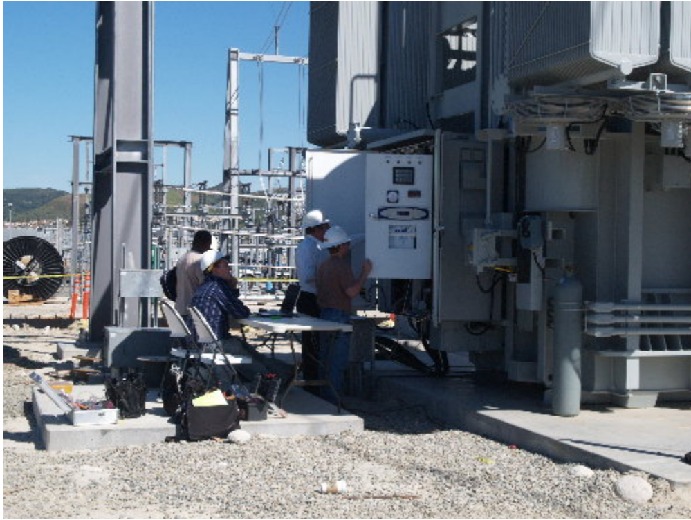
Figure 3 – Testing crews worked to check the various functions of the A-bank transformers prior to operation.
