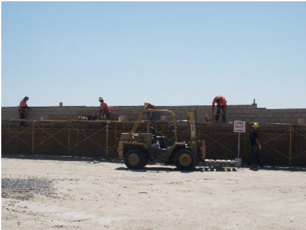
Figure 2 – The Reycon crew worked to set the cap-stones for the block wall.
