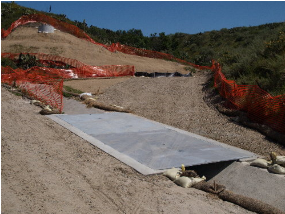
Figure 6 – The permanent plated crossings for the v-ditch on the 66 kV section east of the substation site have been completed.
