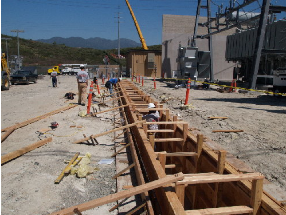
Figure 1 – Crews worked on the wooden form that surrounds the rebar cage for the concrete trench west of MEER #1..
