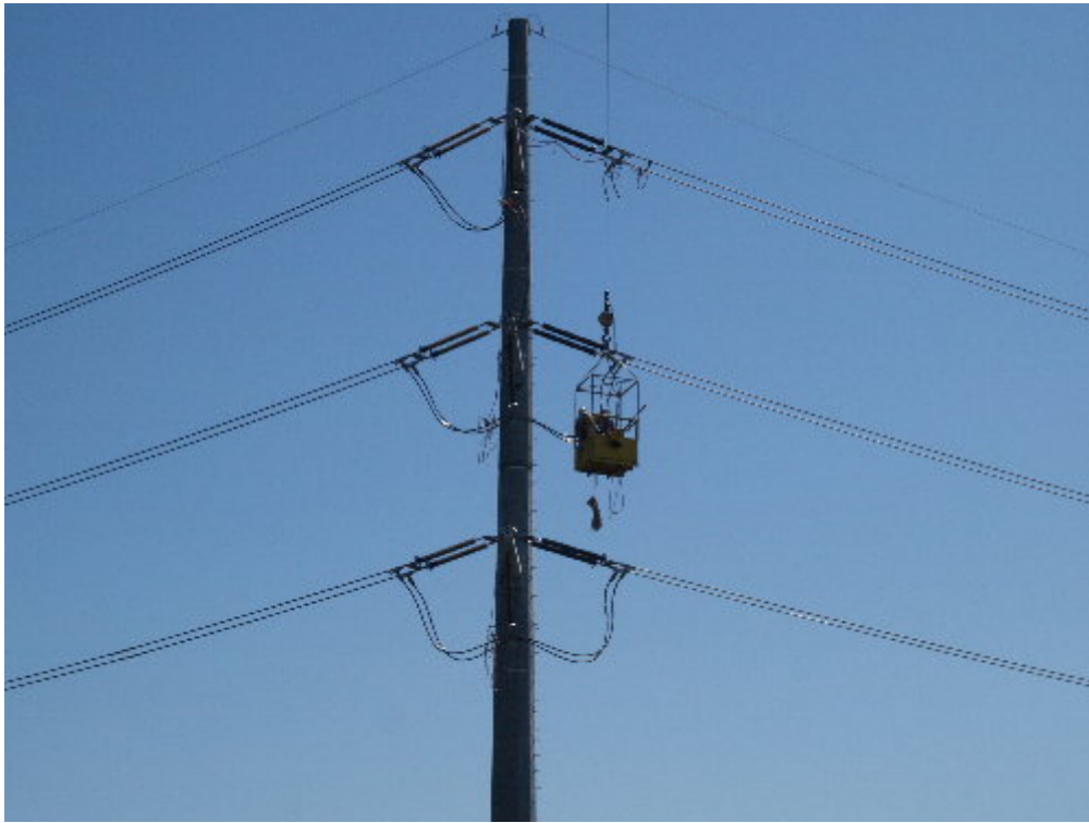
Figure 3 – The SCE transmission line crew worked to connect the jumpers between the two sections of conductor at the turning pole. Note the missing jumper on the top right-hand side of the steel pole.
