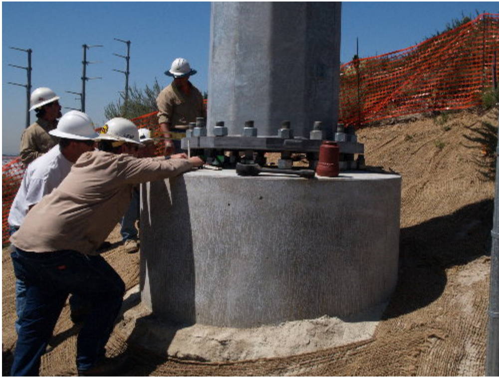
Figure 5 – The crew used the lower bolts to attain the proper angle for the pole.
