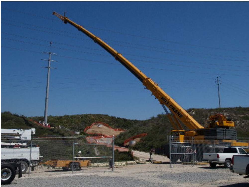
Figure 4 – A larger crew worked with Hill Crane to set a steel pole on a 66 kV foundation.
