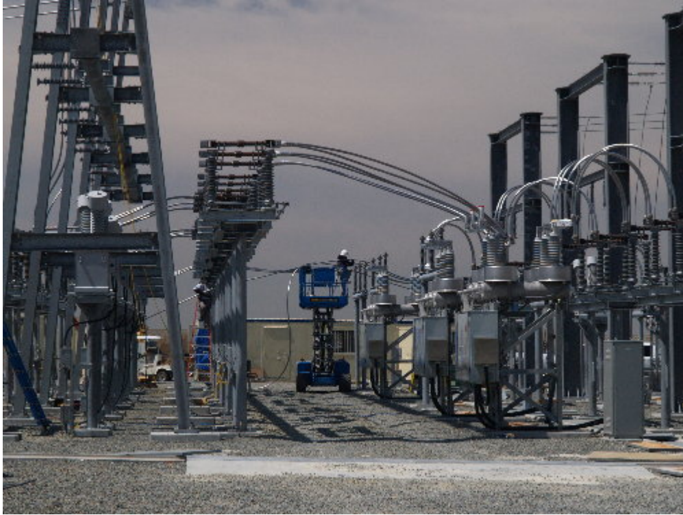
Figure 1 – NRG continued working on the small connections between the various equipment within the 66 kV section of the substation.
