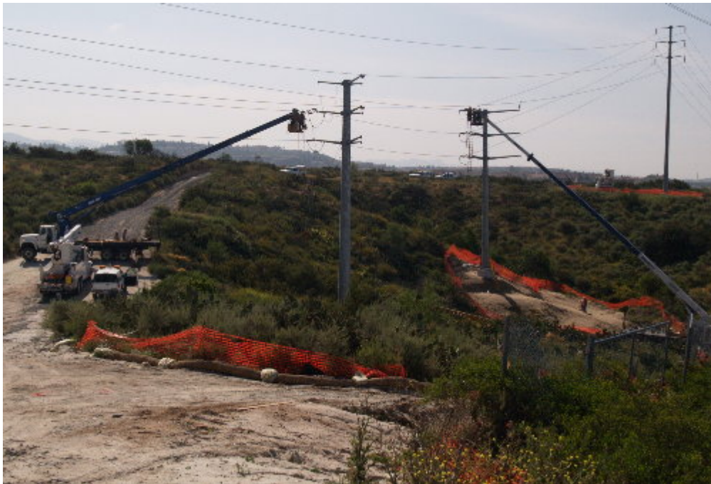
Figure 6 – Crews worked on conductor for the 66 kV line east of the substation during the site visit.
