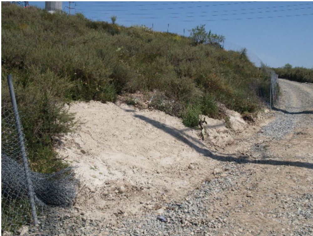
Figure 4 – The crew with American worked to restore sections of the hillside impacted during 220 kV construction.
