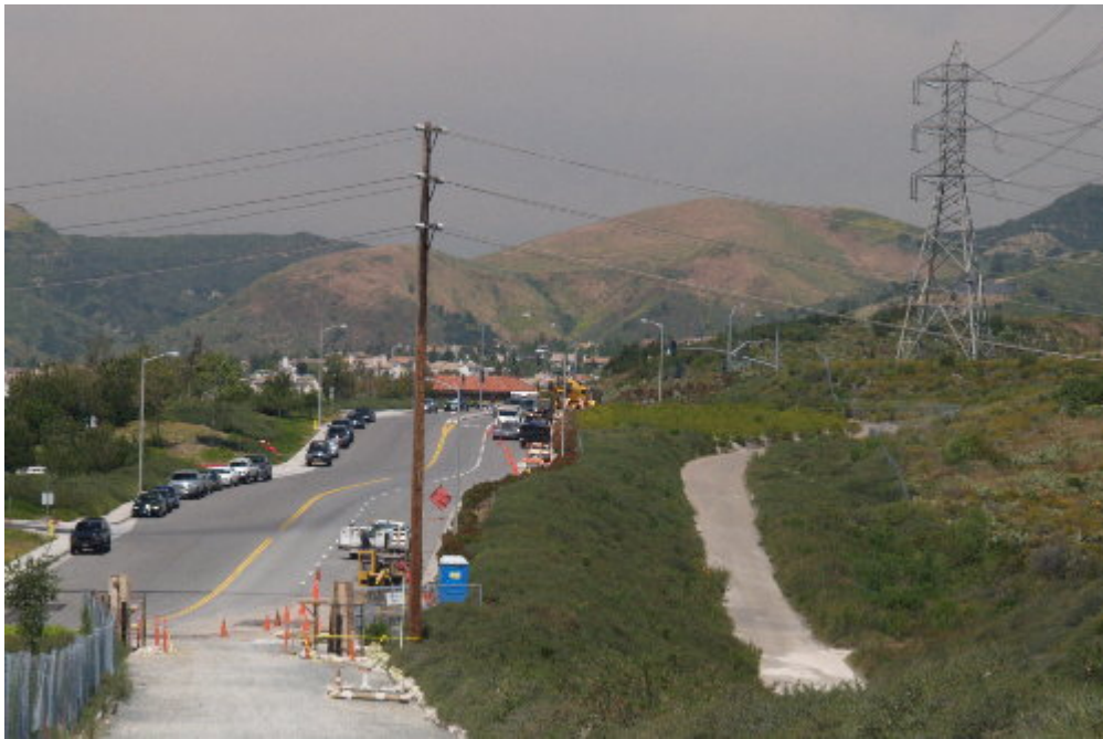
Figure 3 – Crews trenched, placed conduit, and backfilled on Definition Road between the substation entrance and Glenn Ranch Road.
