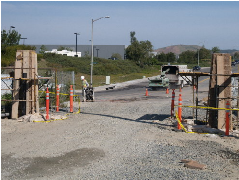
Figure 2 – The Reycon crew has built the block columns at the gate on Definition Road. Note: The truck and chipper are not project-related.
