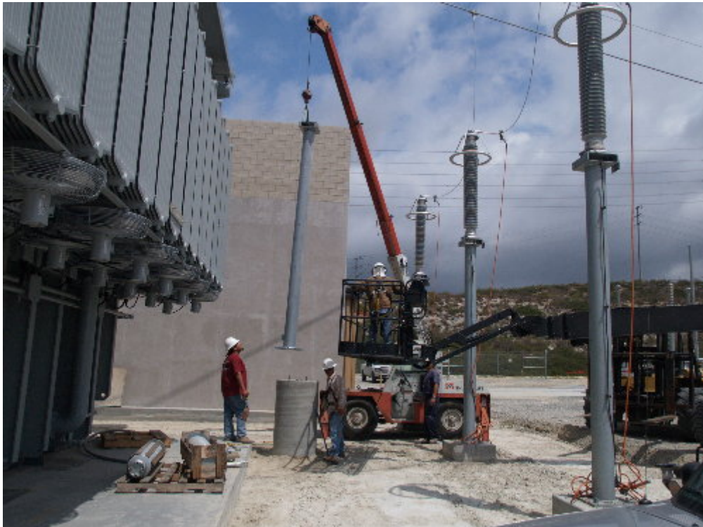
Figure 4 – The new off-set pole was set on the south side of the A-bank transformer.
