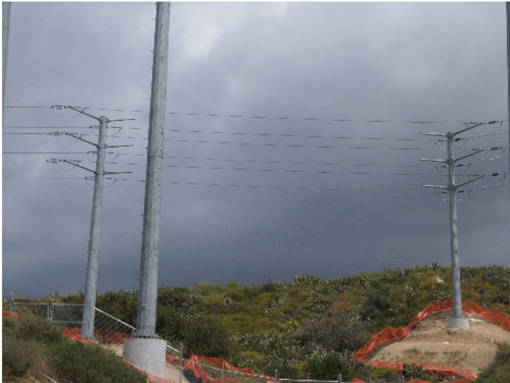
Figure 6 – Crews worked on conductor for the 66 kV line east of the substation prior to the site visit.
