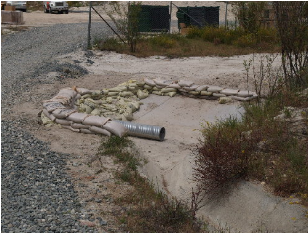
Figure 5 – The American crew cleaned silt out of the concrete lined ditch on the 220 kV right-of-way.
