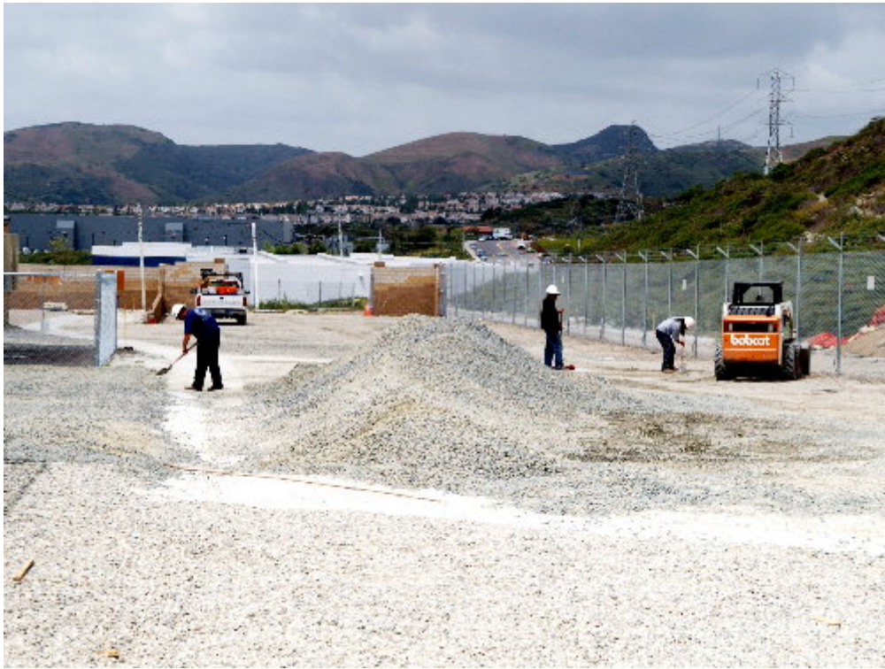
Figure 3 The American crew worked on cleaning out the v-ditches surrounding the substation site.
