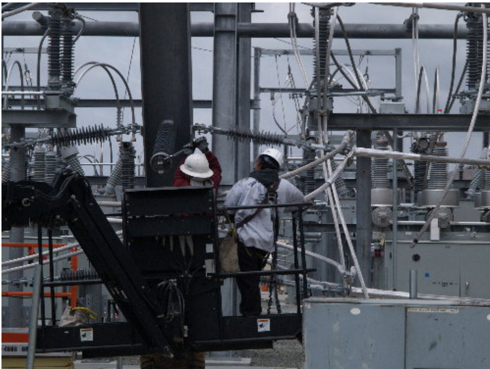
Figure 2 – NRG continued working on the small connections between the various equipment within the 66 kV section of the substation.
