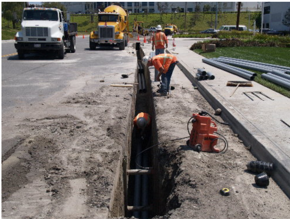
Figure 4 – Arizona Pipeline worked on Ellipse Road, trenching, laying conduit for the 12 kV distribution conductor, and backfilling with slurry.
