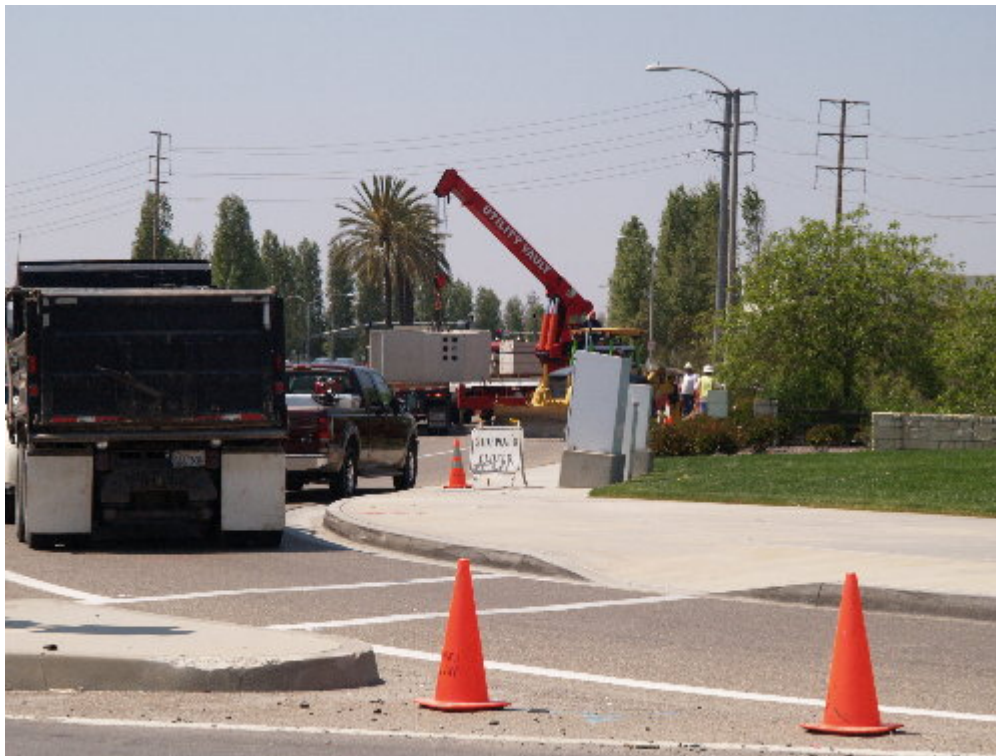
Figure 5 – Arizona Pipeline worked to unload trench vaults on Portola Parkway during the site visit.
