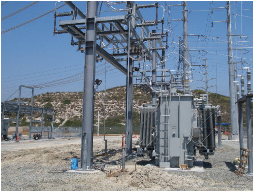
Figure 2 – The manual disconnect switches have been set and the forms for the foundation are ready for concrete.
