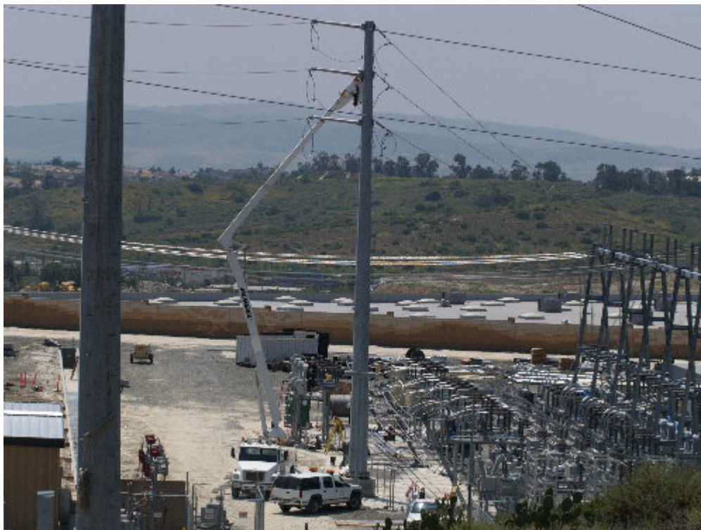
Figure 6 – Crews worked on clipping in conductor between the 66 kV line and the substation during the site visit.
