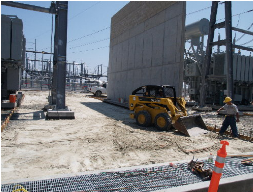
Figure 3 – A crew graded for the concrete pads that will be poured between the various foundations.
