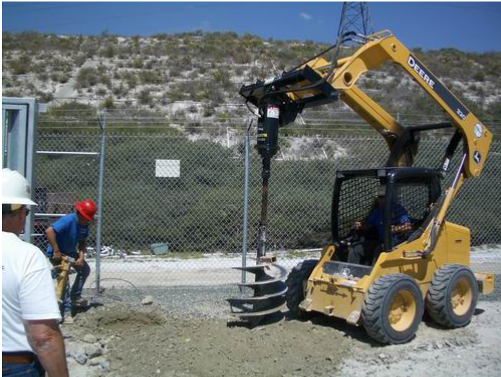
Figure 4 – KGC worked on excavating for the light standard foundations throughout the substation site.
