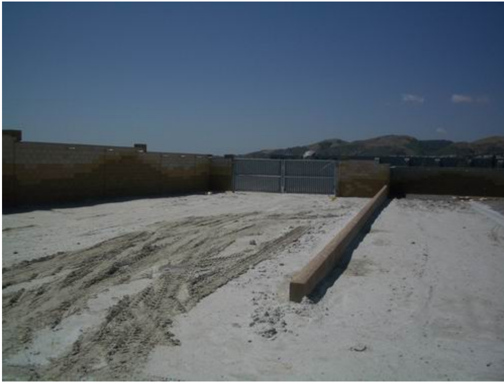
Figure 3 – The main gate and side gate have been set on the previously installed supports.
