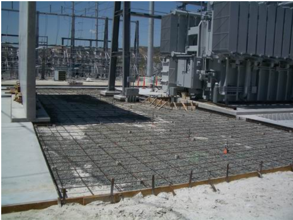
Figure 2 – The forms between the various foundations are ready for concrete. The concrete pads on either side were poured the previous week.
