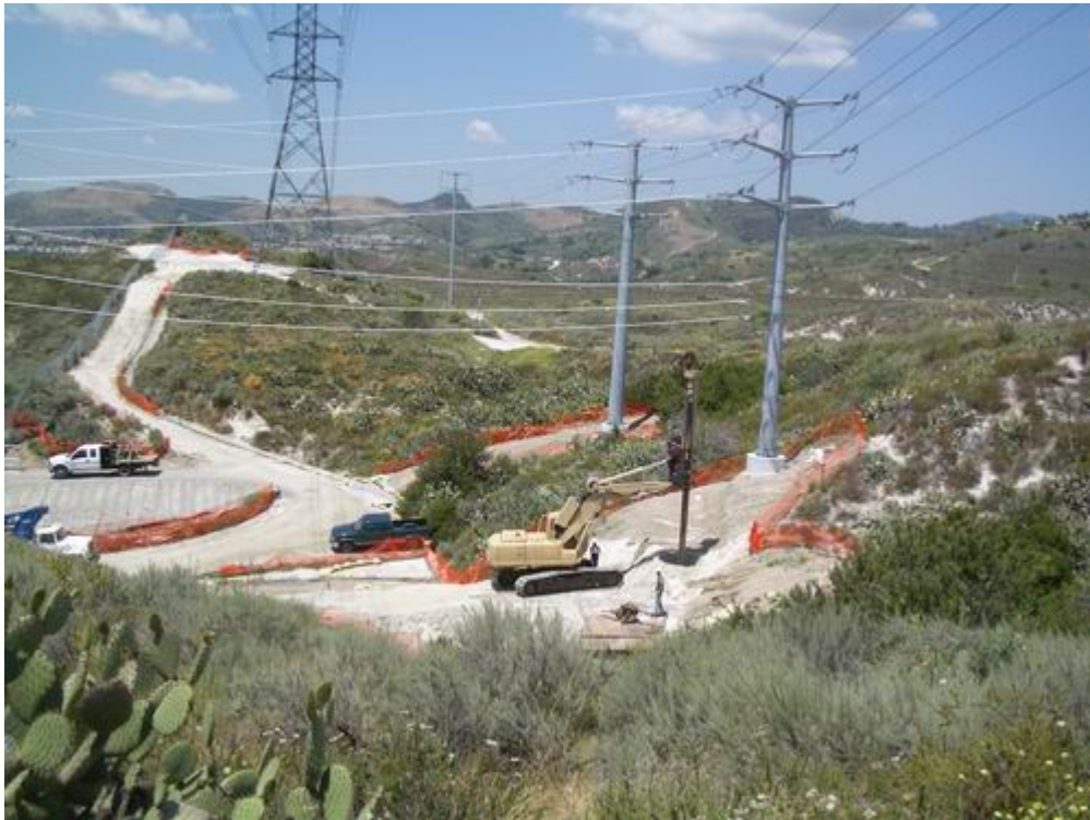
Figure 6 – Crews worked on drilling for the 66 kV H-structure foundations during the site visit.
