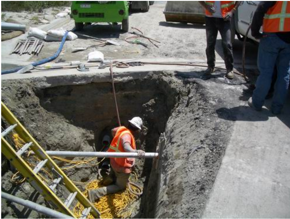
Figure 5 – Arizona Pipeline worked to clean out the previously placed conduit between Definition Road and the substation site.
