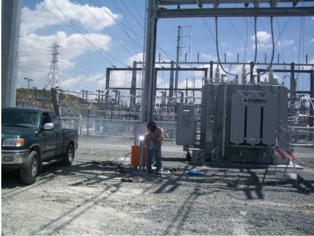
Figure 1 – The foundations for the manual disconnect switches have been poured and a welder worked to complete the installation.
