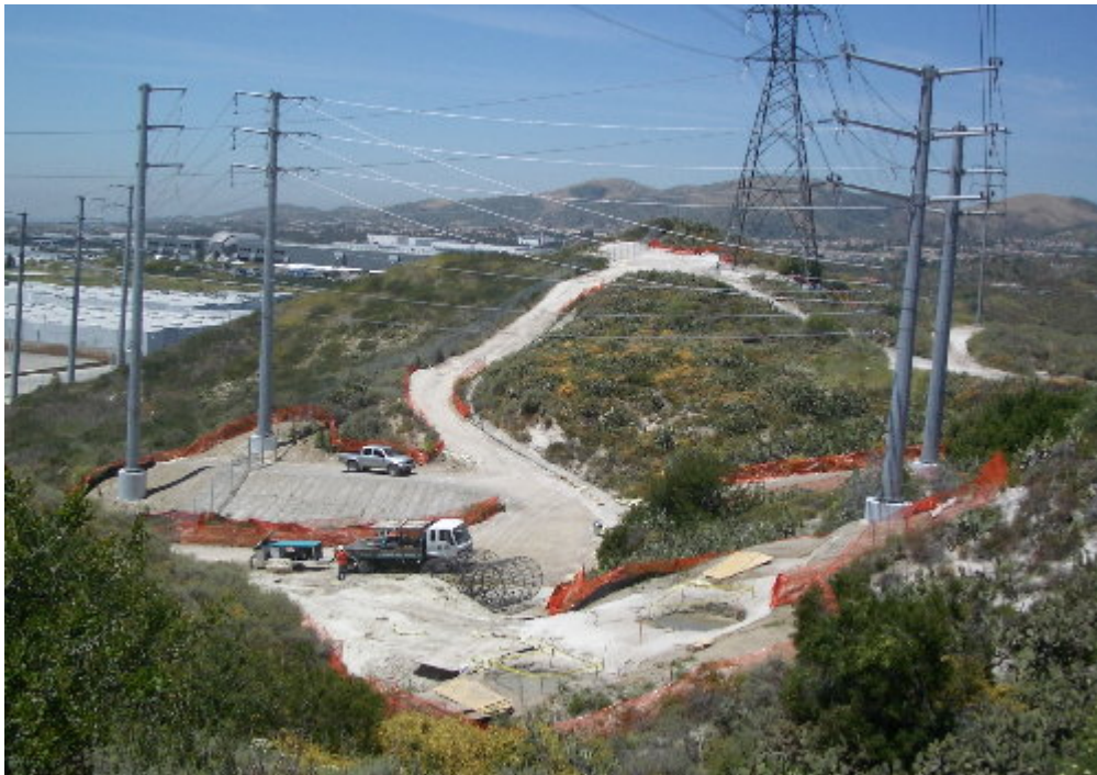
Figure 6 – Crews prepared the rebar cages for the 66 kV H-structure foundations during the site visit.
