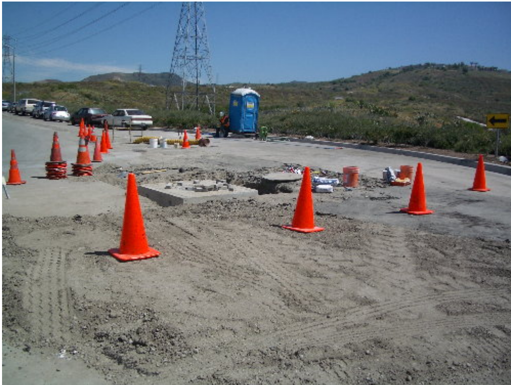
Figure 4 – Arizona Pipeline set a vault for the 12 kV conduit on Definition Road at the substation site.
