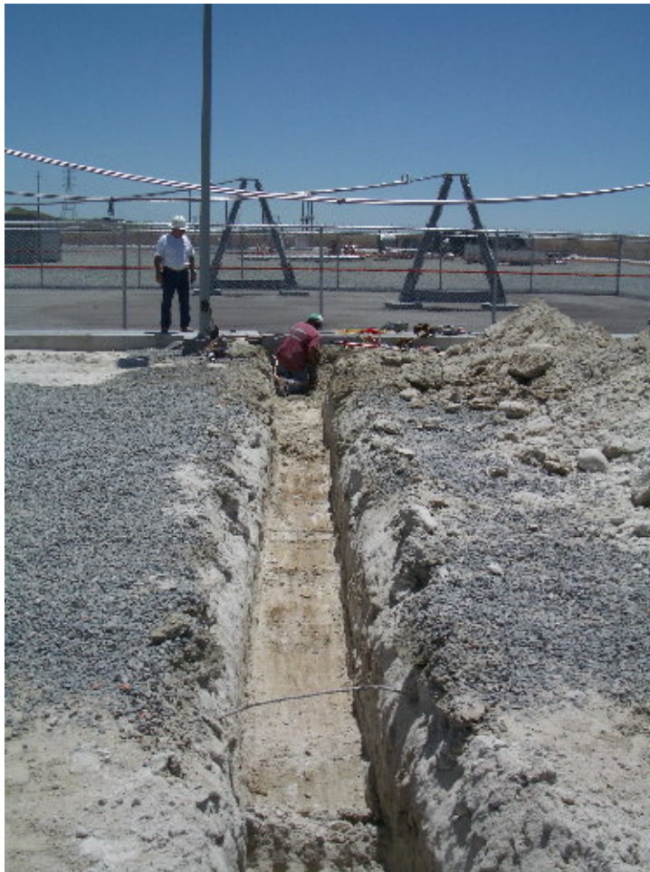
Figure 2 – KGC excavated a trench for future expansion and tie it into the existing pre-formed concrete trench adjacent to the 220 kV fence.
