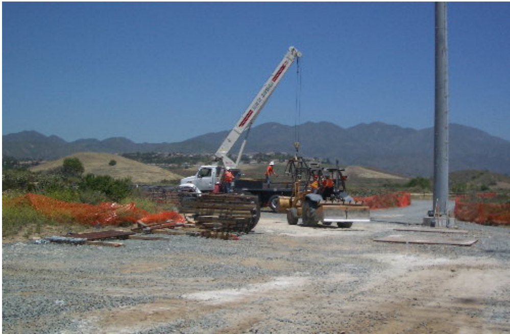
Figure 5 – Arizona Pipeline crews unloaded equipment for setting the rebar cages and anchor bolts for the 66 kV H-structure above the substation site.
