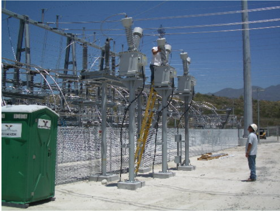
Figure 1 – NRG crews worked on adjusting the insulators and other equipment during the site visit.
