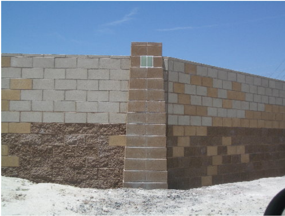
Figure 3 – Reycon started installing the glass blocks in the pilasters on the block wall.
