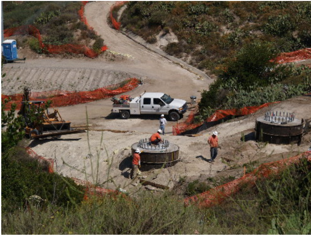
Figure 3 – The forms for the new foundations for Structure 13 were removed during the site visit.
