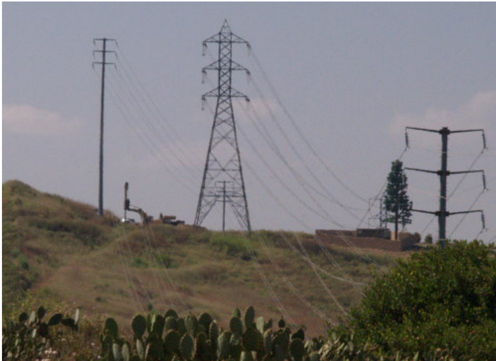
Figure 4 – Work continued on the foundations for Structure 10, in the City of Mission Viejo.
