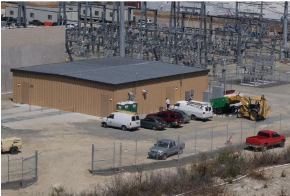
Figure 2 – An emergency generator was set outside MEER #1.
