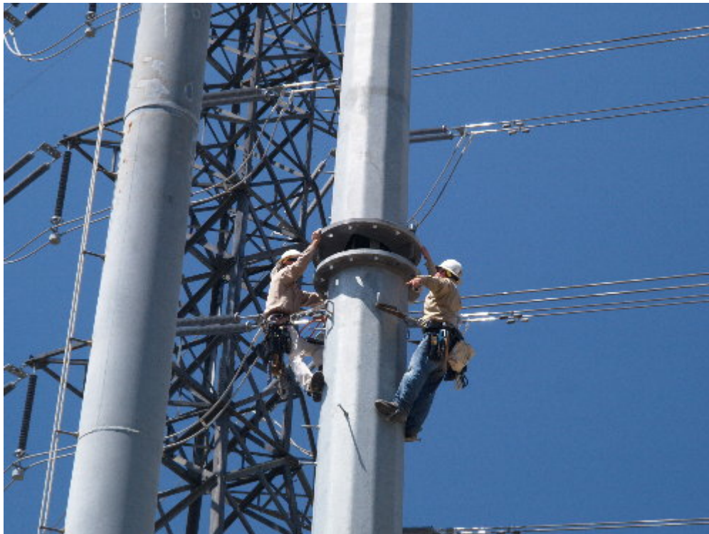
Figure 6 – Workers helped guide the upper section of the east pole for H-Structure 12 and then bolted the sections together.
