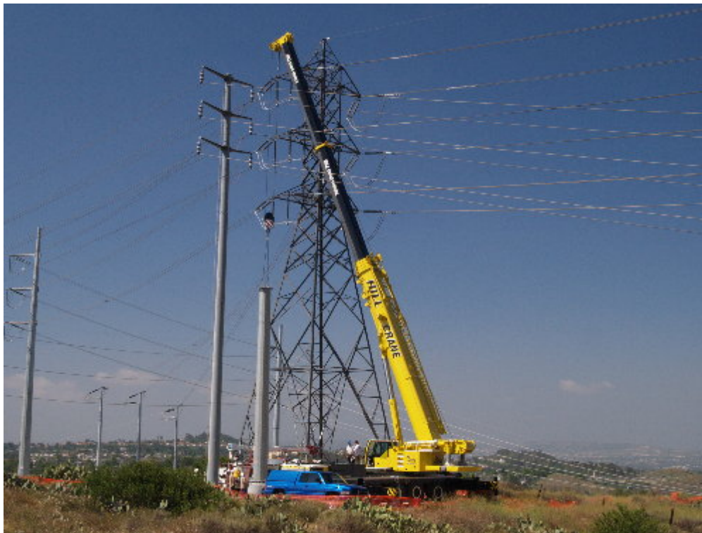
Figure 5 – A large mobile crane was set up on-site to assist in raising the steel sections of H-Structure 12.
