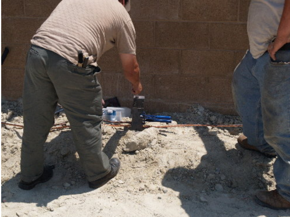
Figure 3 – A small crew worked to repair the grounding grid within the substation site.
