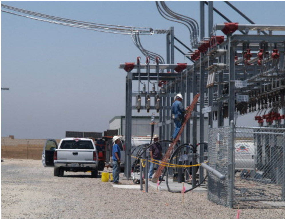
Figure 1 – A Hampton Tedder crew worked to connect the underground cables to the racks; thereby connecting the substation site to the SCE distribution system.
