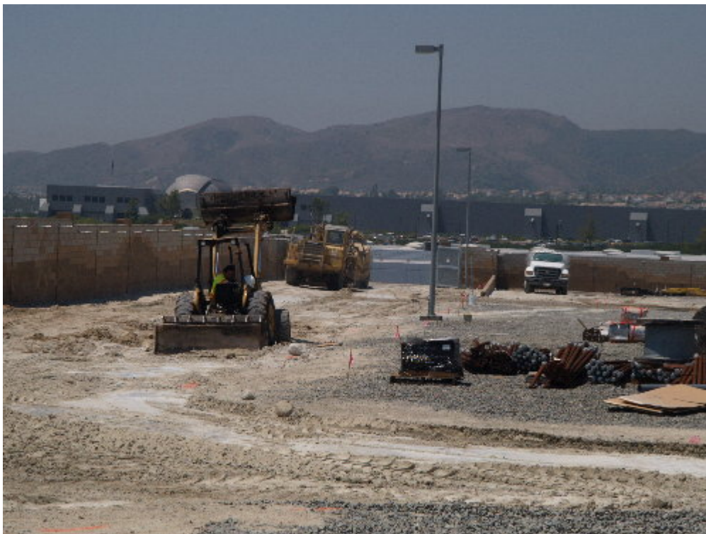
Figure 2 – The paving contractor worked to grade the road sites prior to paving.
