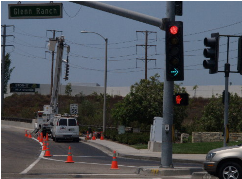
Figure 1 – A Hampton Tedder crew worked in the underground vault on Portola Parkway, connecting the substation site to the SCE distribution system.
