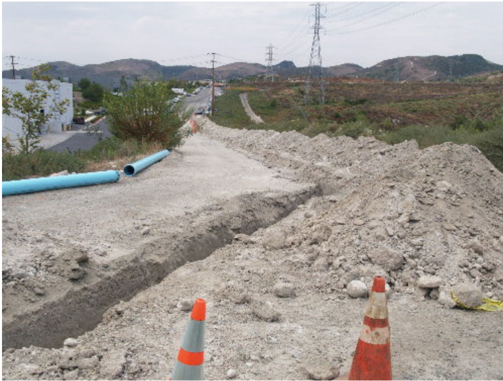
Figure 3 – A subcontractor worked to trench through the hard ground and lay the water supply line for the fire control system.
