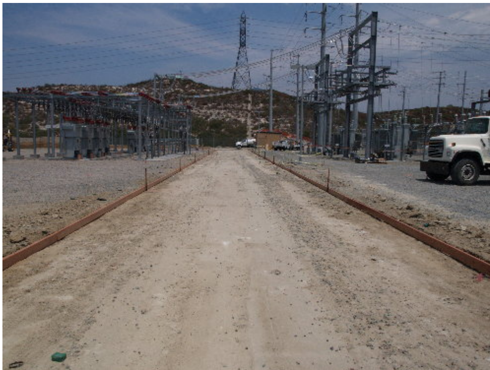
Figure 2 – The paving contractor finished rough grading of the substation roadway prior to paving.
