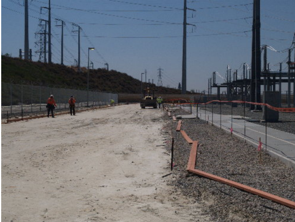
Figure 1 – The paving contractor crew worked on installing the borders for the substation roadway prior to paving.
