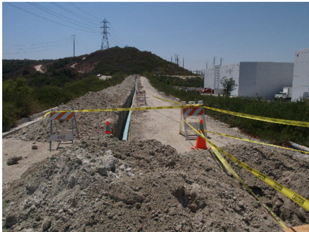
Figure 2 – A subcontractor trenched along the access road to lay the water supply line for the fire control system.
