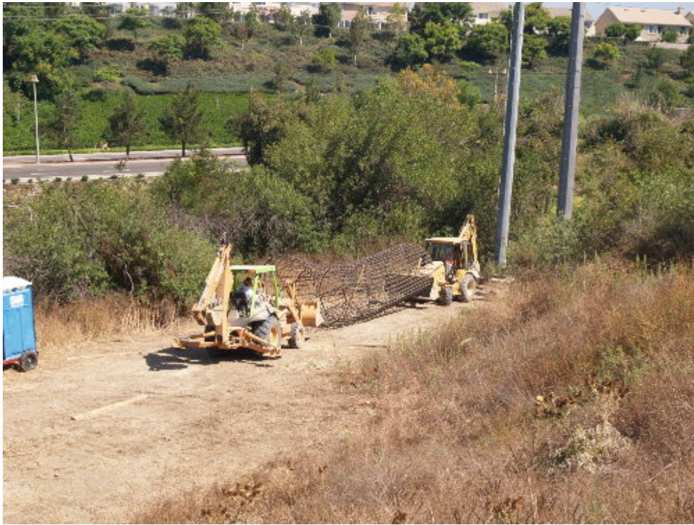
Figure 5 – The re-bar cage was moved to the excavation at H-Structure 1 (at Chiquita Substation).
