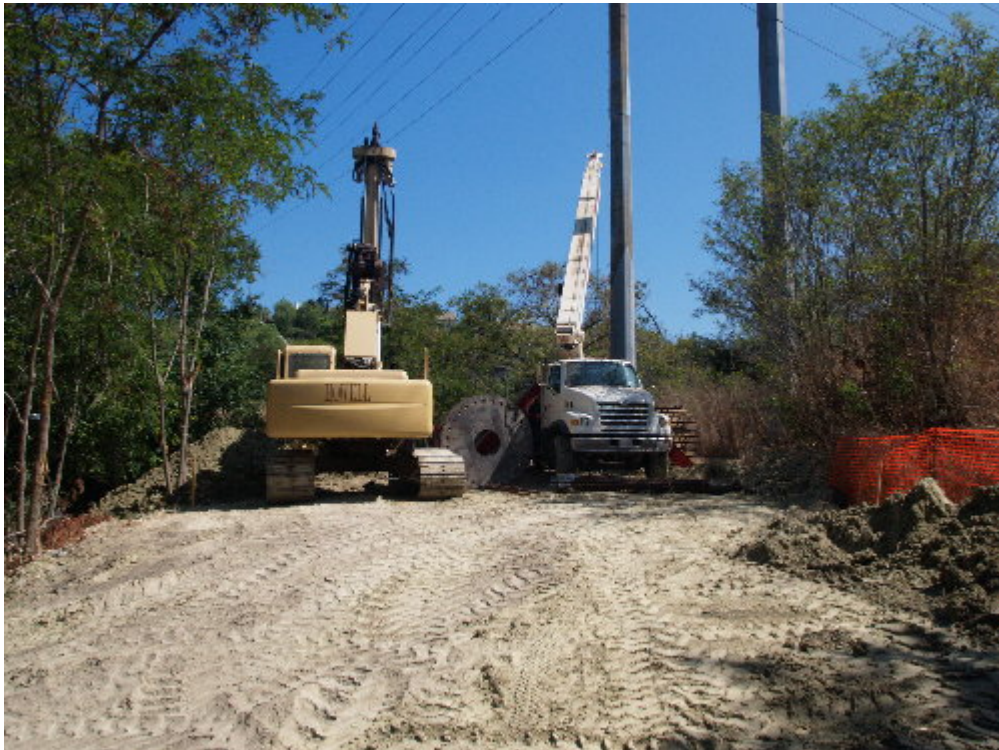
Figure 4 – The drilling crew worked to prepare H-Structure 1 (at Chiquita Substation) for the concrete pour.
