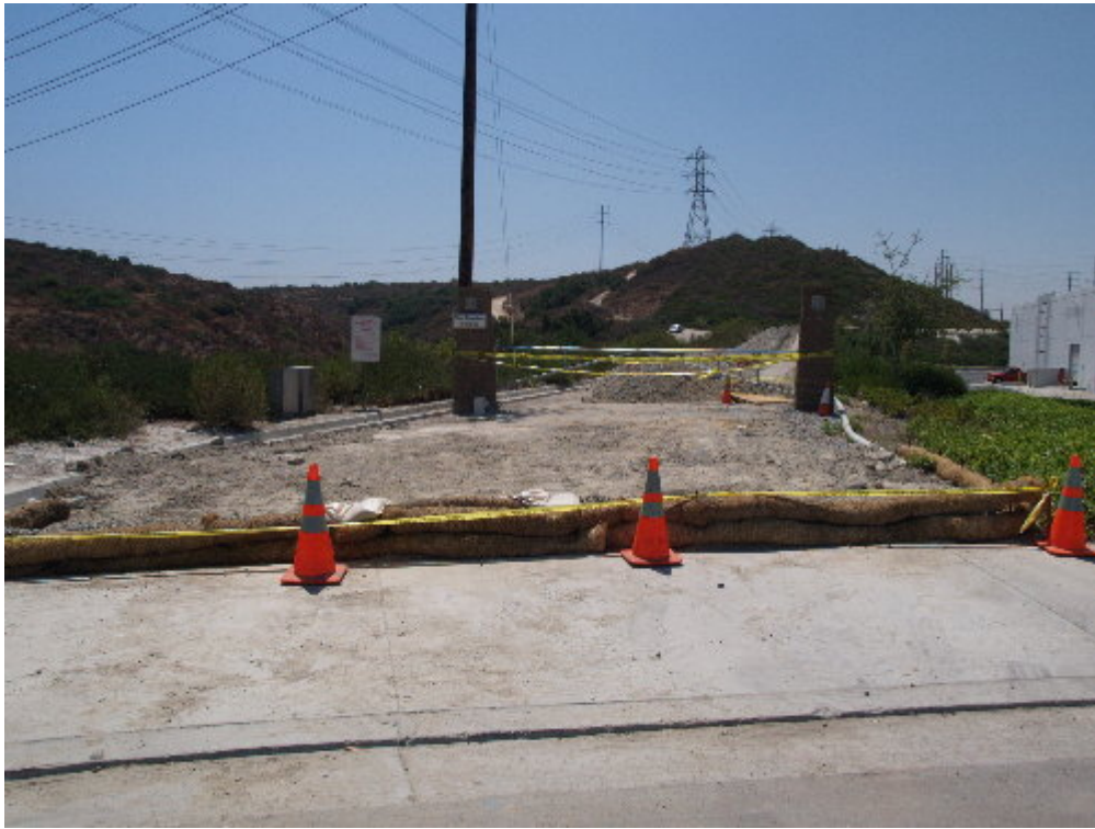
Figure 3 – BMPs were installed to prevent sediment from entering the public roadway and adjacent storm drains.
