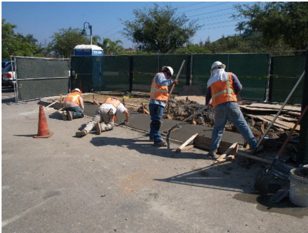
Figure 4 – An Arizona Pipeline crew worked on the curb access at Olympiad Park.
