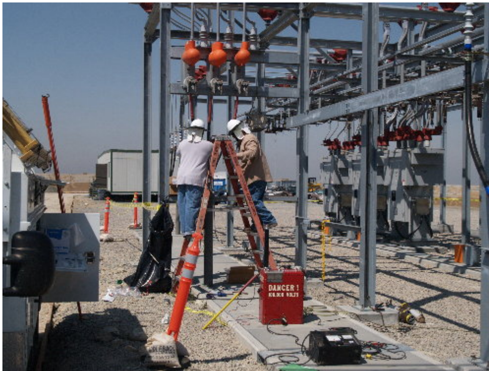
Figure 3 – An SCE crew worked to connect station light and power during the site visit.
