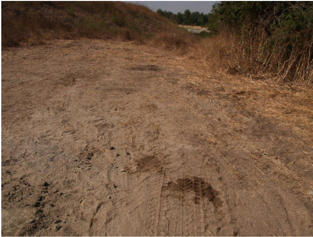
Figure 5 – The small oil spill at the Chiquita Substation will be addressed by Arizona Pipeline.
