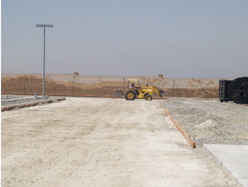
Figure 1 – The paving contractor crew worked placing rock on the borders for the substation roadway prior to paving.
