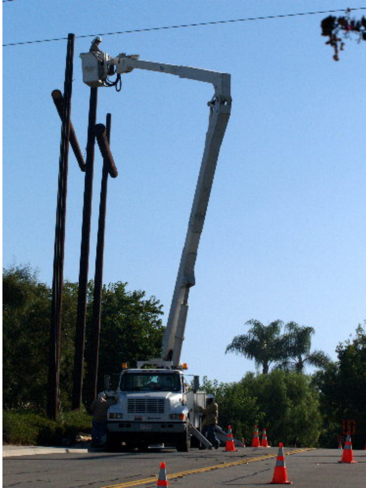
Figure 1 – The transmission line crew used a truck mounted man-lift and crane to raise the timber for extending the guard structure at La Barca.
