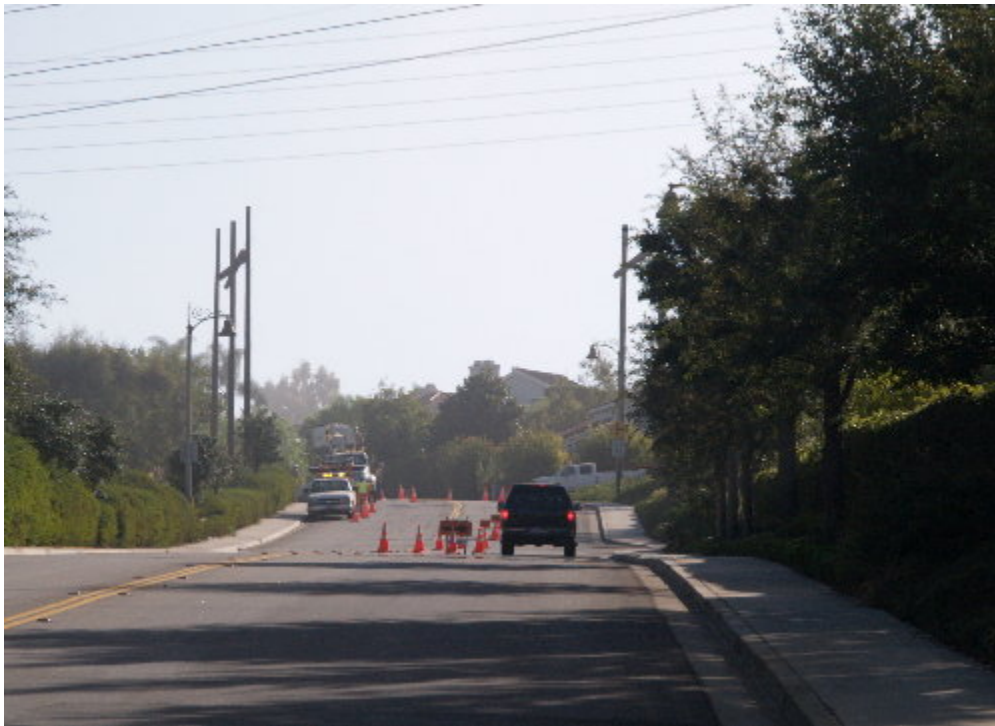
Figure 2 – Although only the curb was used during extension of the guard structure, traffic controls were placed to protect both the crews and the public.
