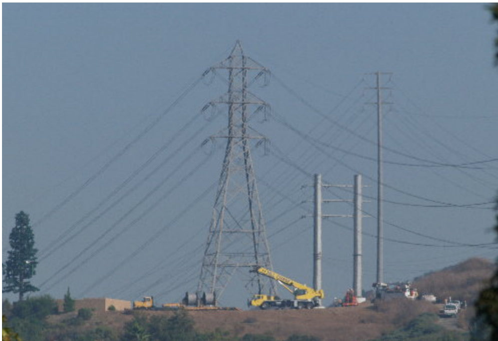
Figure 3 – Reels of conductor and stringing equipment was set at H-Structure 10 to prepare for pulling conductor between Structure 10 and Structure 7.
