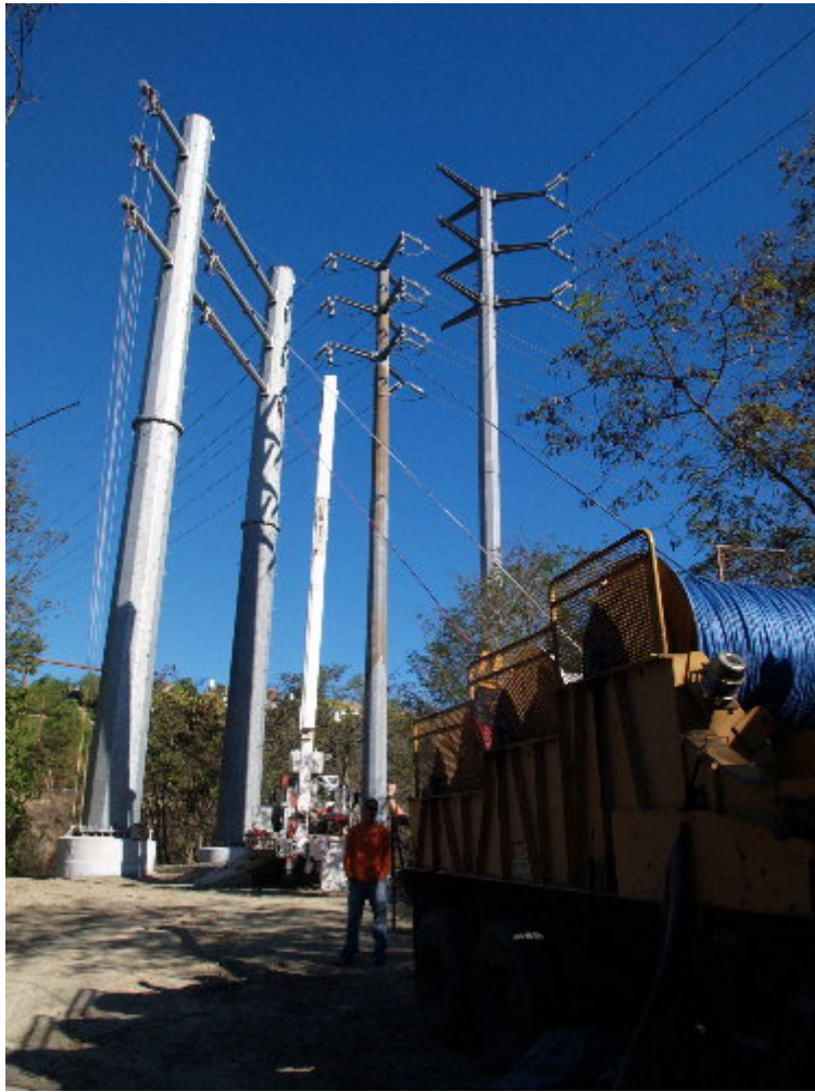
Figure 2 – The SCE transmission line crew worked to pull conductor between Structures 5 and 1. Structure 1 is adjacent to the Chiquita Substation.
