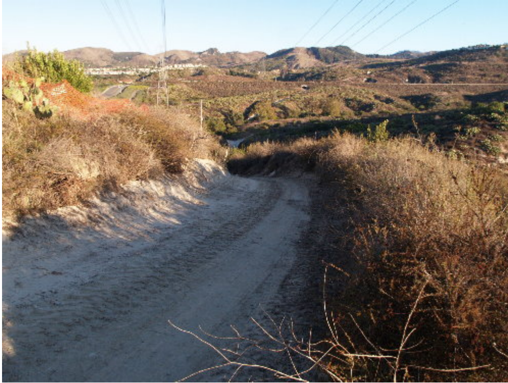
Figure 1 – A crew unrelated to the Viejo System Project installed communication conduit in the SCE right-of-way above the Viejo Substation. This disturbance will require stabilization prior to rainfall.
