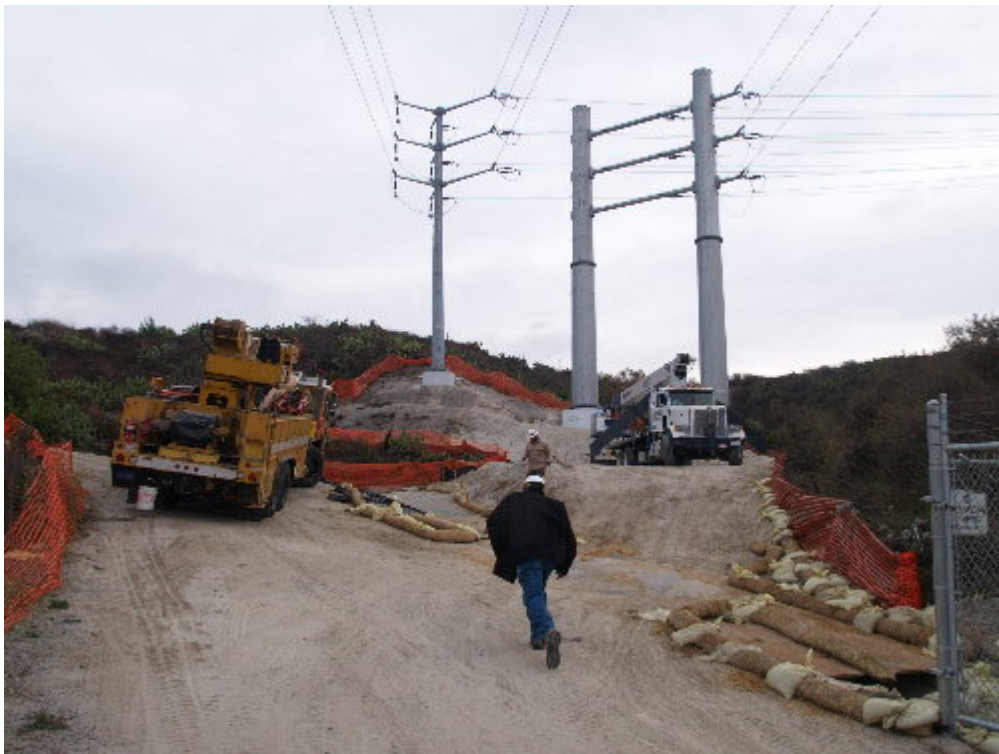
Figure 2 – A SCE transmission crew worked at Structure 13, on the right-of-way above the Viejo Substation, preparing to move conductor to the center position between Structure 13 and the substation.
