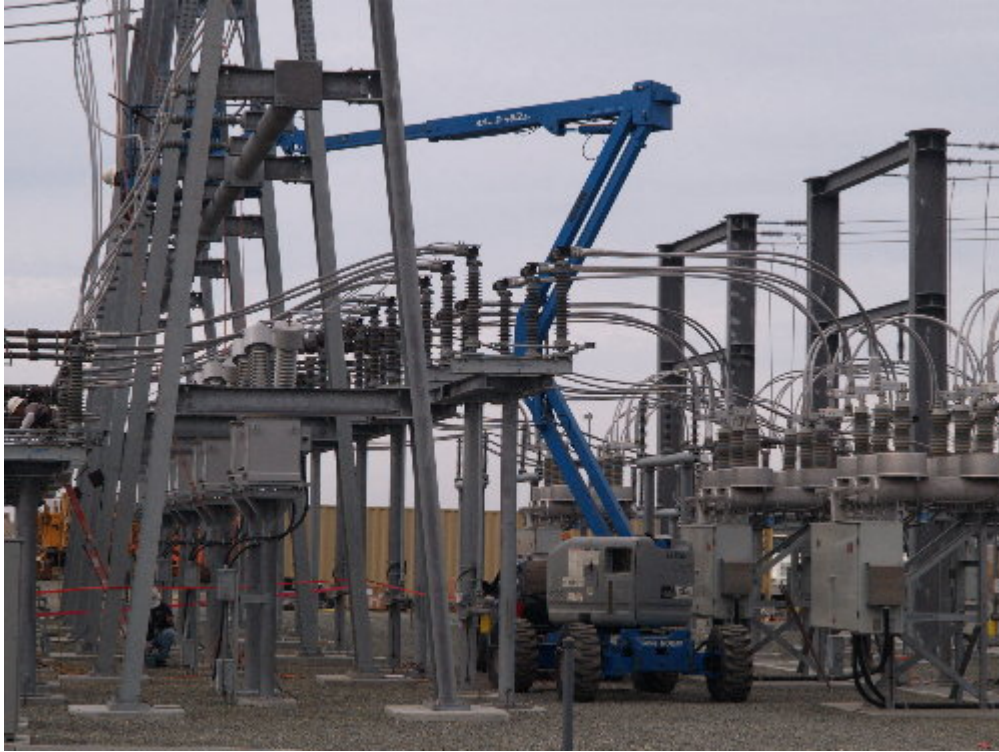
Figure 1 – A small crew worked within the Viejo Substation during the stringing activities.
