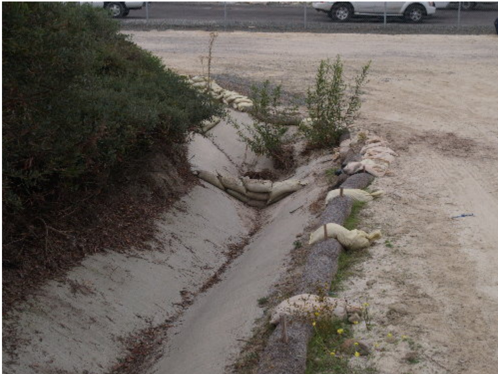
Figure 4 – The BMPs in and around the Viejo Substation were cleaned out in preparation for the predicted rainfall.
