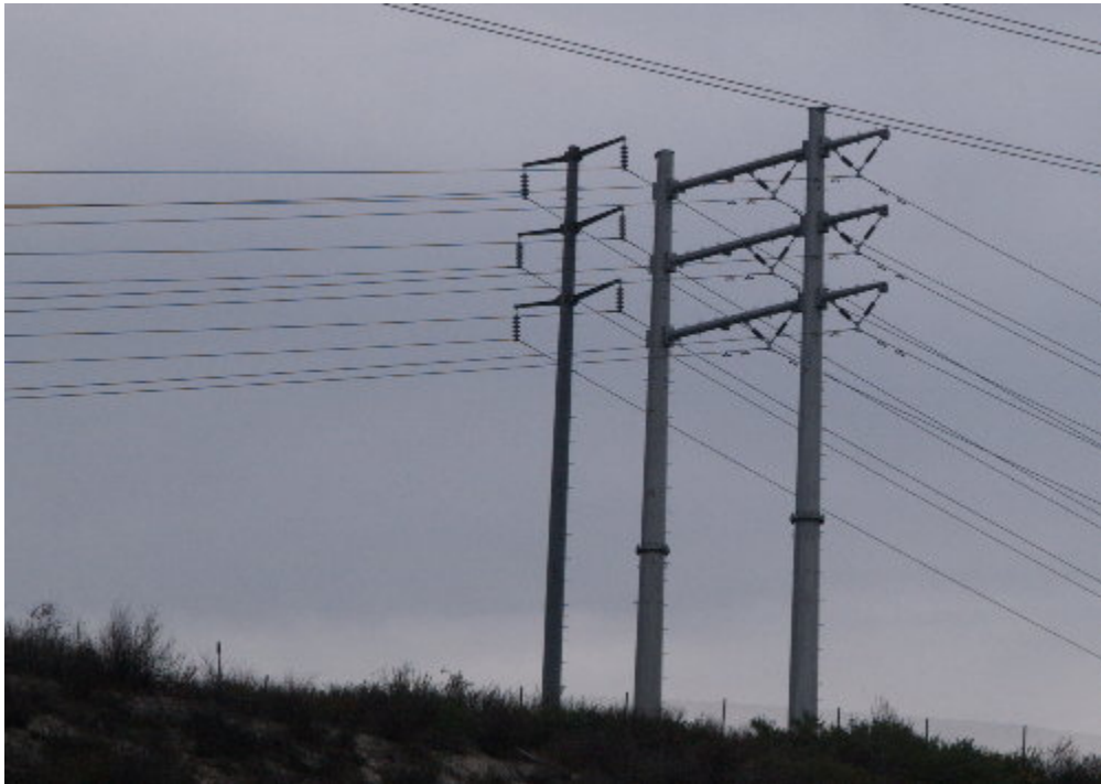
Figure 3 – Conductor can be seen in one of the center positions of Structure 12. The H-Structures are designed to accommodate two circuits in the center position; however, only one will be placed at this time.
