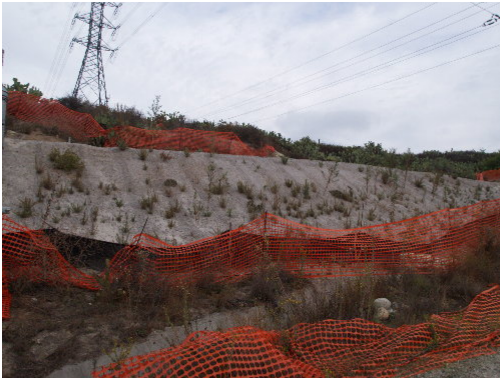
Figure 5 – Some recruitment of native species was observed on the slopes of the structure pads above the Viejo Substation.
