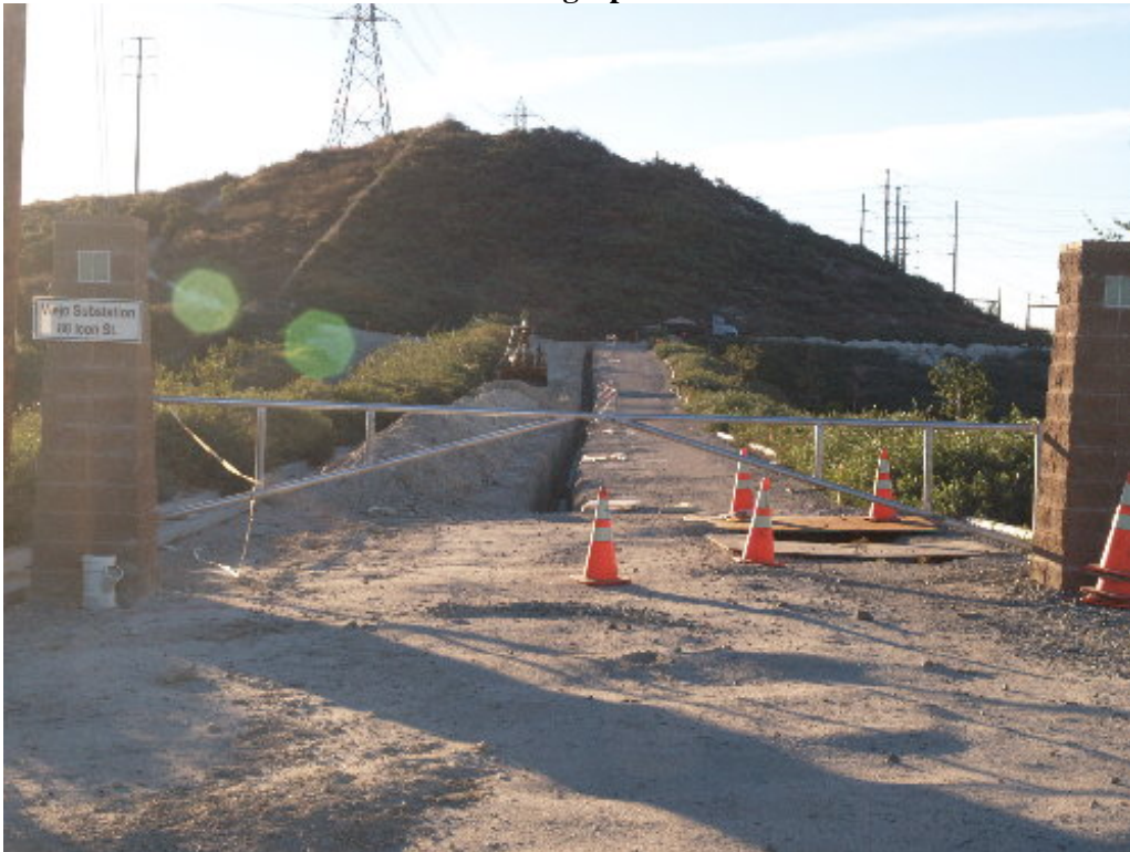
Figure 1 – The company installing a communication line along the main access road removed the spoils from the water line in order to trench along the east side of the line.
