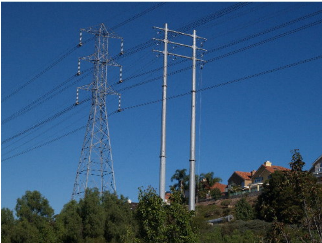
Figure 4 – The east arm has been installed on the H-Structures now that many of the old 66 kV steel poles have been removed. Note the old steel pole on the ground.
