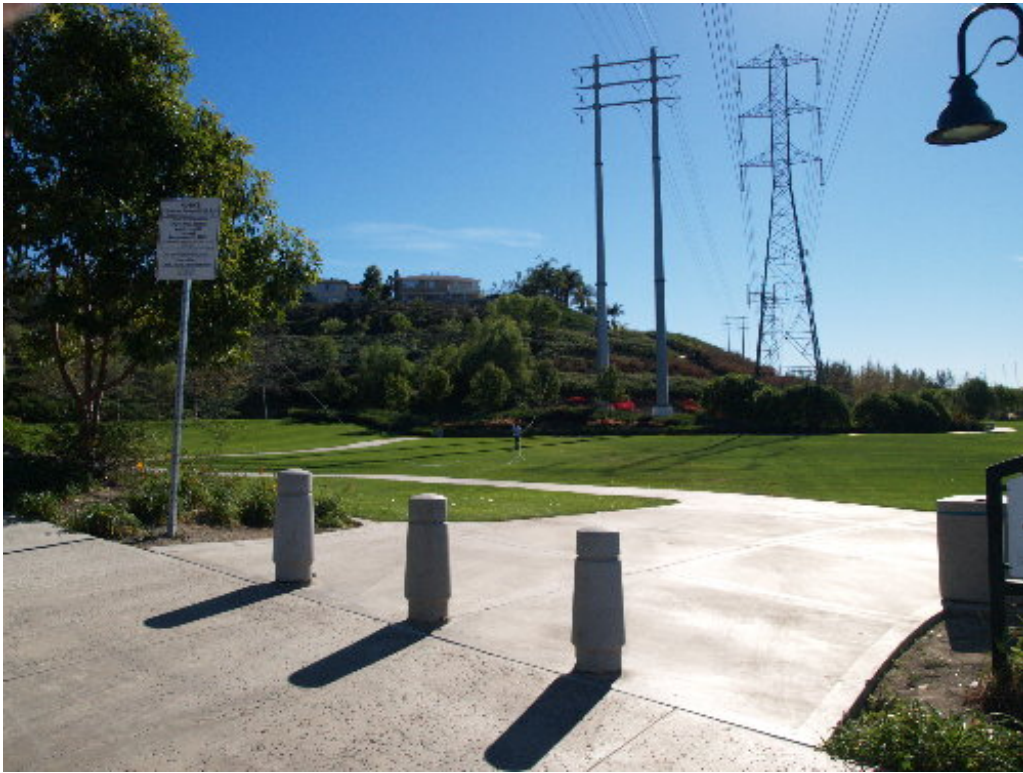
Figure 5 – SCE worked within Olympiad Park pulling sock line in preparation for stringing the new conductor on the east arm of the H-Structures.
