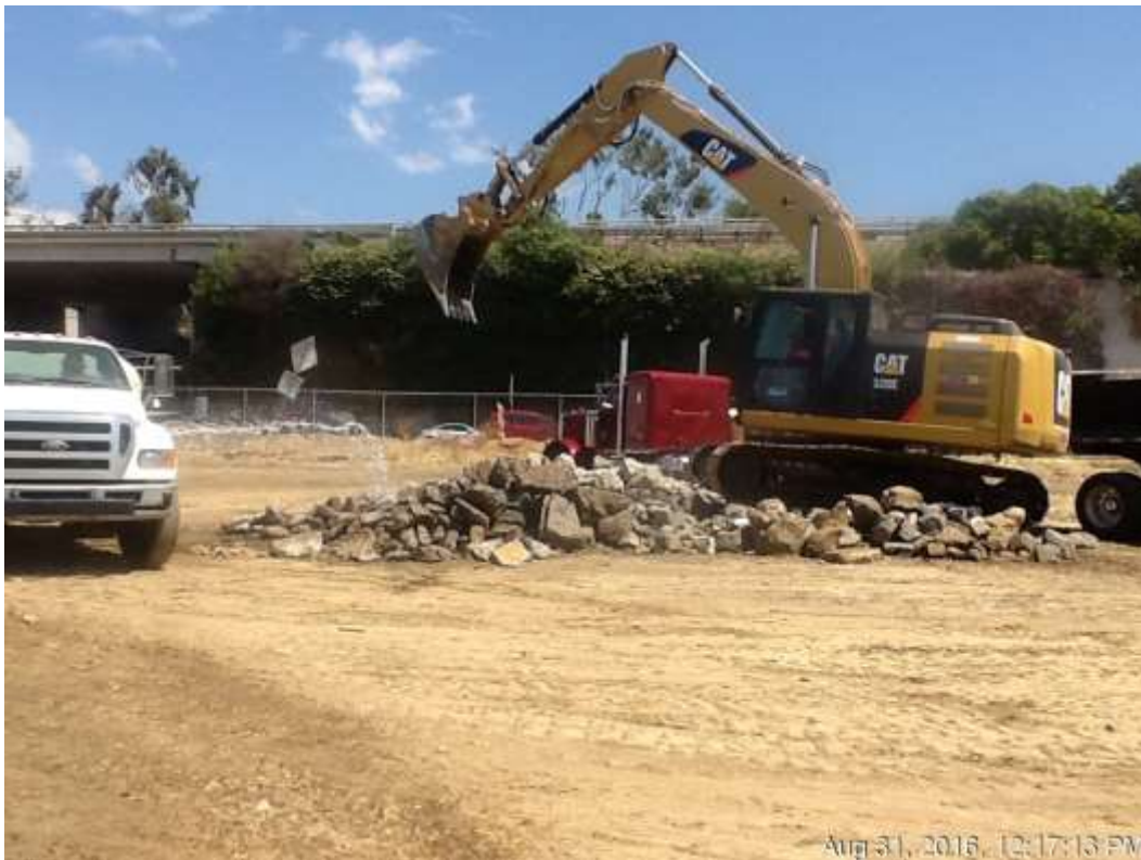
Figure 6 – Water was applied to the debris pile to minimize dust from the demolition and hauling operations.
