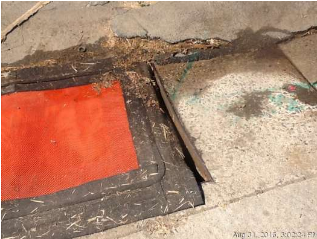
Figure 5 – The hydrant water flowed into a storm drain along Vine Street and also flowed onto the substation site.
