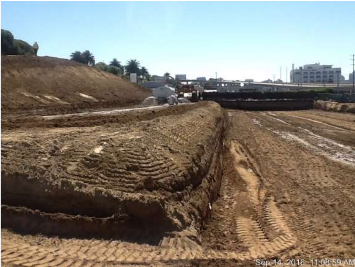
Figure 3 – Watering for dust control and compaction is taking place on a regular basis.
