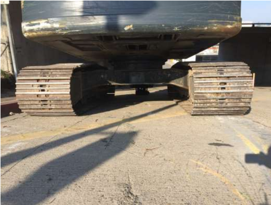
Figure 3 – The CPUC EM found an excavator used by NPL crews stored after work without the necessary drip pan.
