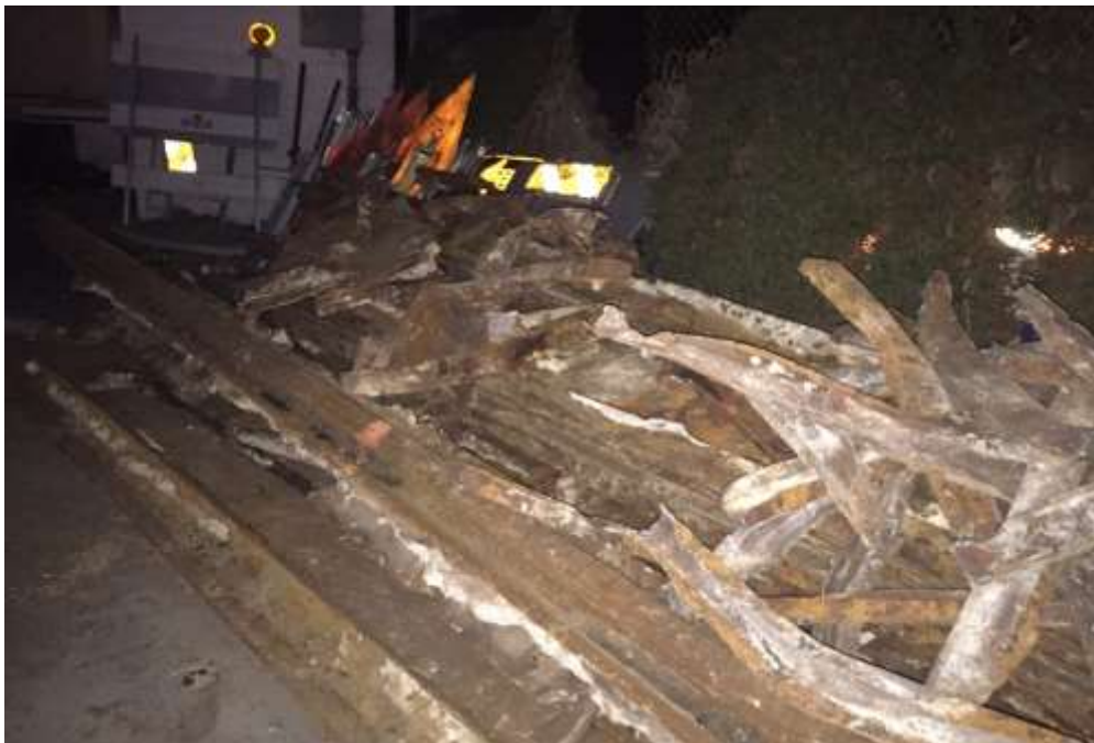
Figure 2 – NPL crews working along Kettner Boulevard salvaged abandoned rail segments from the trench and vault excavations. These sections are put aside for recycling and for collection by the Pacific Southwest Railway Museum.
