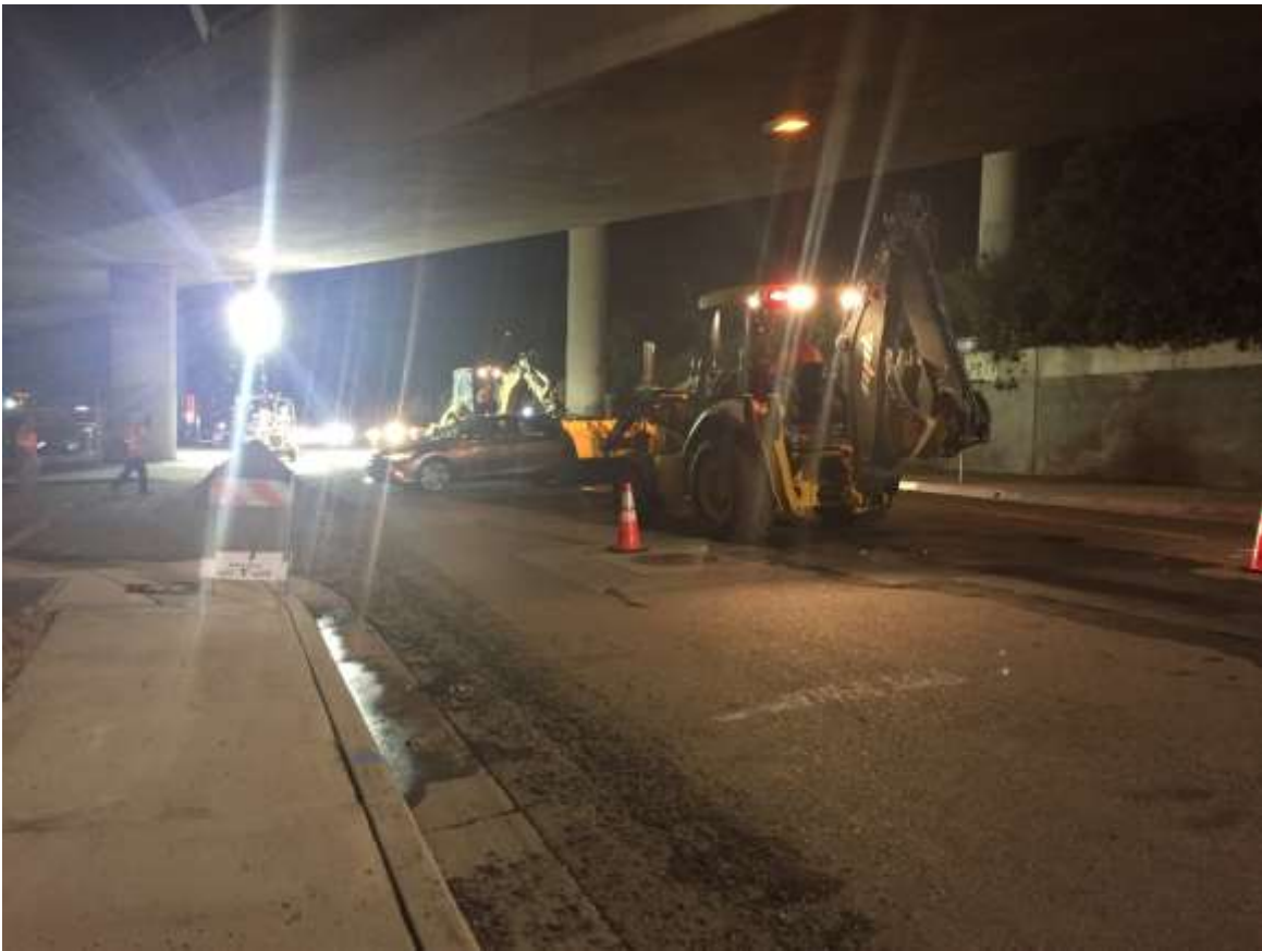
Figure 3 – Traffic control and construction activity the night of October 5 at the intersection of Kettner and W. Redwood Street. A vehicle drove through the work area to access a parking lot on W. Redwood Street. Open access to Redwood Street was not provided, inconsistent with Traffic Control Permits.
