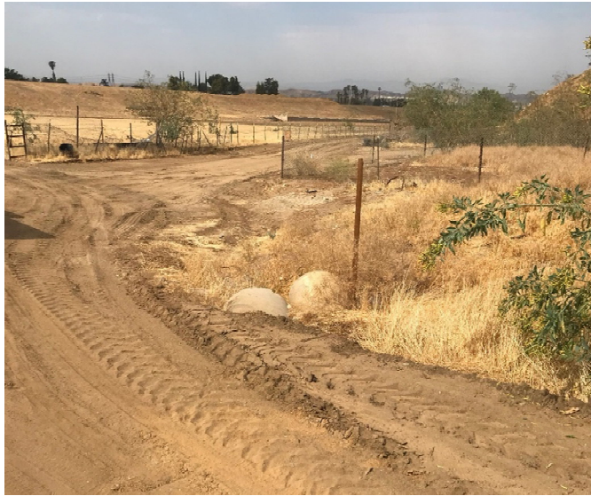
Photo 2. Concrete pipe culvert exit on west side of dirt access road, which conveys flow under the road to the southwest immediately to sheet flow upon exiting. Photo facing southwest.
