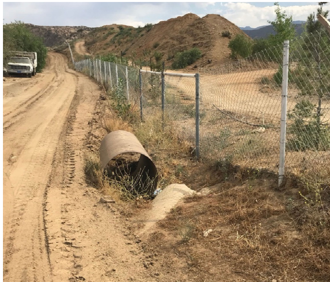
Photo 1. Concrete pipe culvert on the east side of dirt access road, which conveys sheet flow from the northeast dirt roads under the road. Photo facing north.
