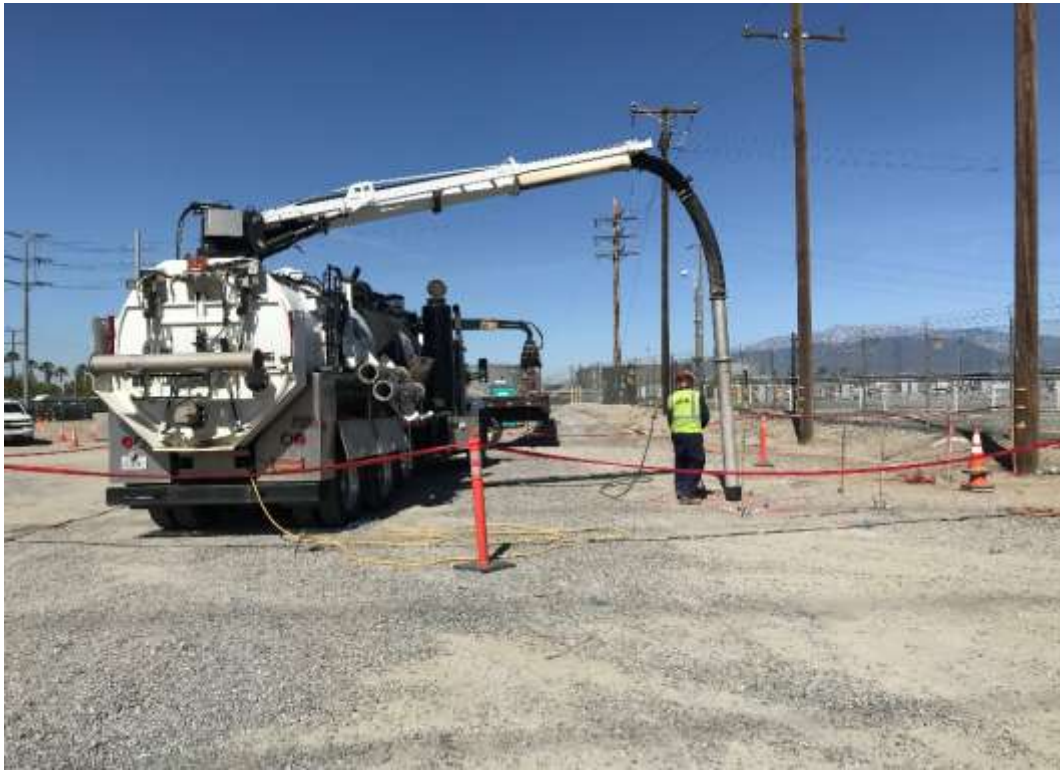
Photo 5 – Potholing for utilities ahead of TSP excavation associated with Tennessee Relocation (April 18, 2018).
