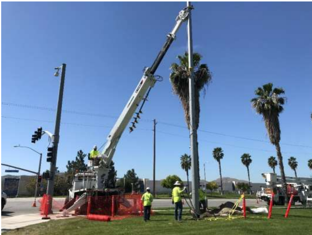
Photo 6 – Installing LWTSP associated with the Tennessee Relocation along San Bernardino Avenue (April 18, 2018).
