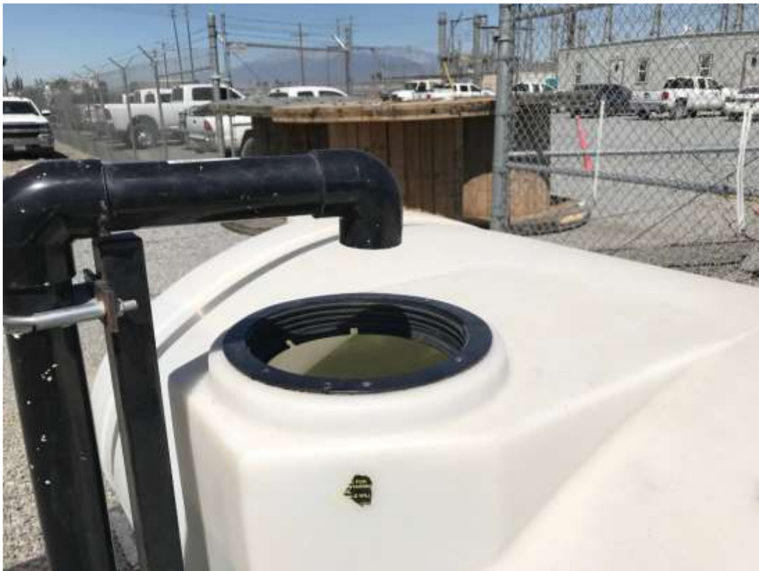
Photo 8 – Portable water tank observed uncovered (April 17, 2018).
