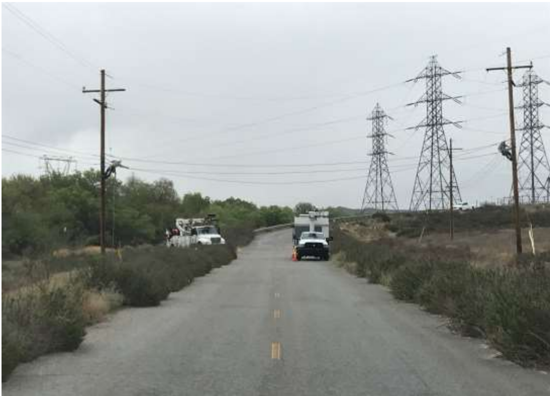
Photo 7 – SCE crews installing fiber along the access road to El Casco Substation (April 19, 2018).
