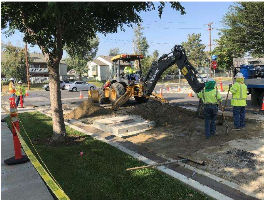
Photo 6 – Trenching for underground conduit installation along Iowa Street for Tennessee Relocation (June 21, 2018).
