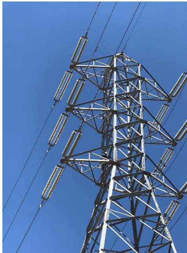
Photo 8 – Barnard lineman removing inactive raven nest along Segment 4 in coordination with biological monitor on the ground. Per requirements of the NBMP, a photo is being captured and relayed to monitor to confirm the nest does not contain viable eggs or chicks prior to removal (June 19, 2018).
