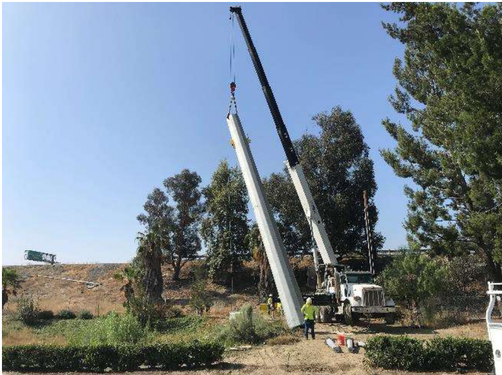
Photo 5 – Erecting TSP at Bryn Mawr Avenue along Interstate 10 for Timoteo Relocation (June 21, 2018).
