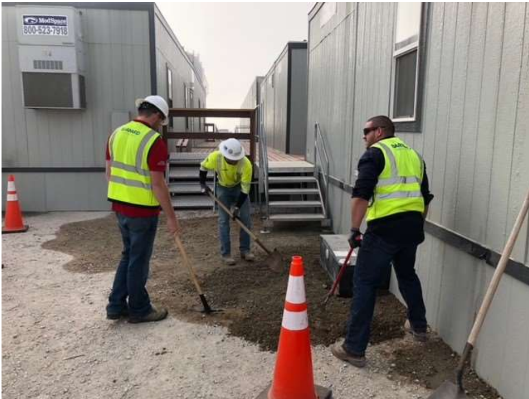
Photo 3 – Removing contaminated topsoil due to spill at Poultry MY (photo courtesy of SCE) (June 21, 2018).
