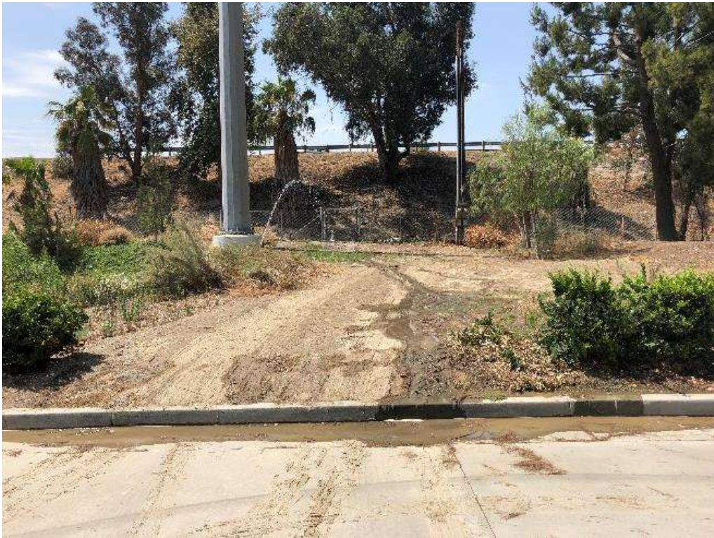
Photo 6 – Broken sprinkler head resulting in minor offsite sedimentation at Bryn Mawr Avenue and Interstate 10 (July 12, 2018).
