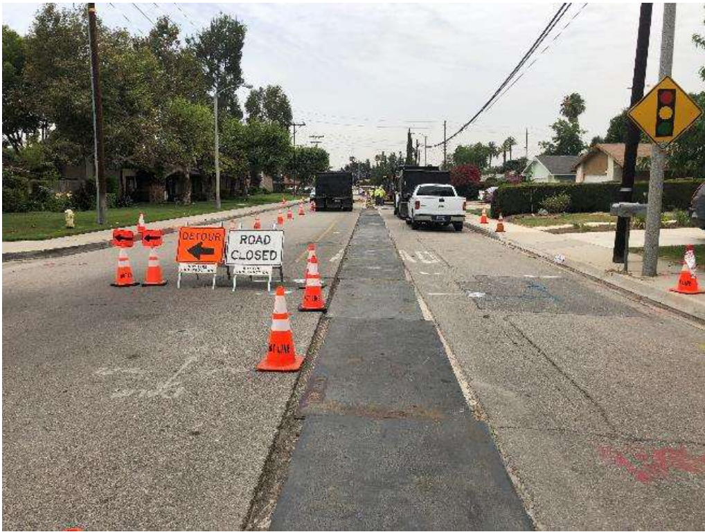
Photo 5 – Ineffective traffic control established along Mission Road for the Dental and Intern Circuits distribution work (July 10, 2018).
