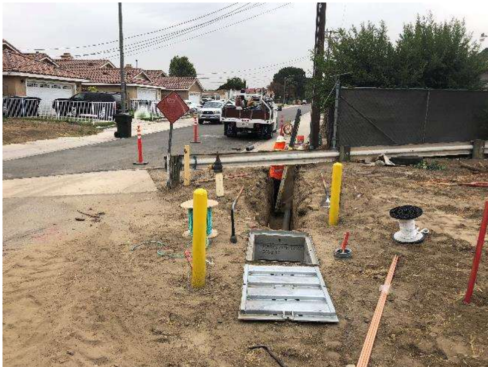
Photo 2 – Working in trench next to riser pole for Juanita Reconstructor distribution (July 10, 2018).
