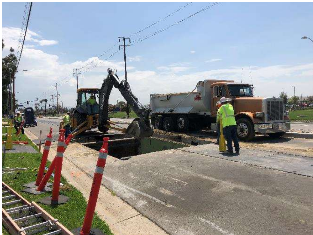
Photo 4 – Excavation of new vault location along Redlands Boulevard for the Timoteo Relocation subtransmission work (July 12, 2018).
