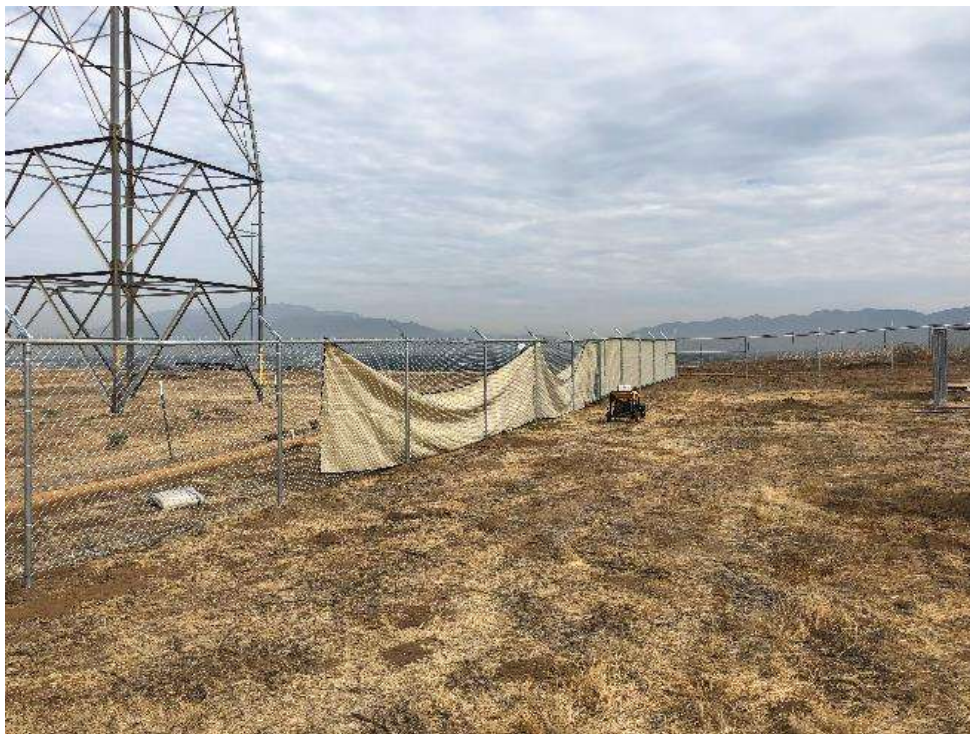
Photo 2 – Cold Smoke Fencing crew installing privacy screening at Grand Terrace MY (July 30, 2018).
