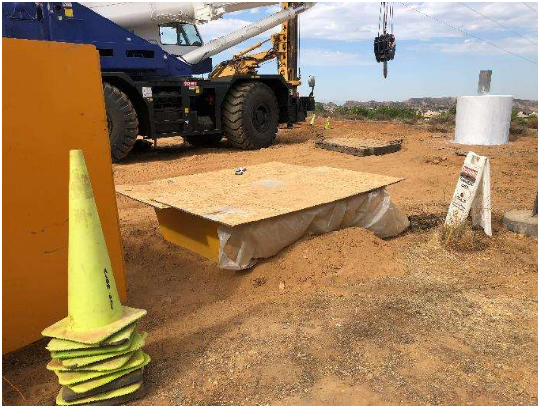
Photo 7 – Inadequate secondary containment for concrete washout pan at Tower Site 4X48, Segment 4 transmission (July 31, 2018).
