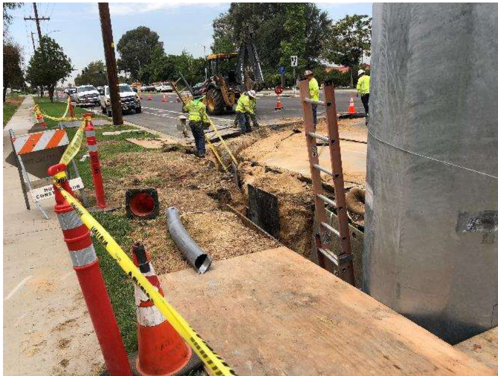
Photo 4 – Underground work being performed at Iowa Street and Barton Road along Tennessee Relocation (July 31, 2018).
