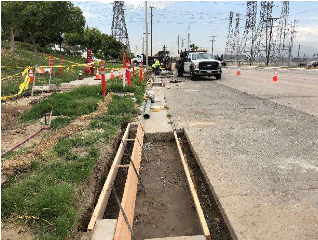
Photo 5 – Curb and gutter repairs along San Bernardino Avenue for Timoteo Relocation (July 31, 2018).
