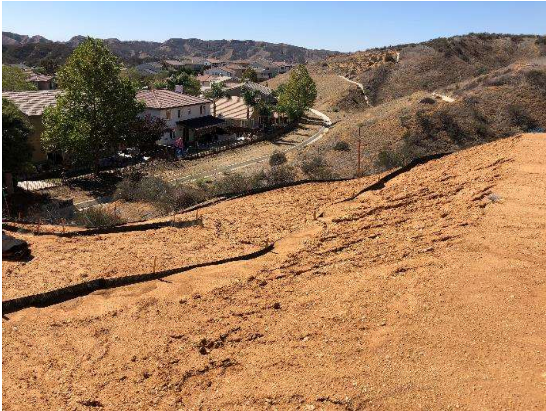
Photo 10 – Accumulated sediment behind BMPs at Site 4X53, Segment 4 (October 15, 2018).
