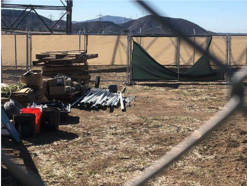
Photo 1 – Fence posts without adequate covering at the Grand Terrace MY (October 18, 2018).
