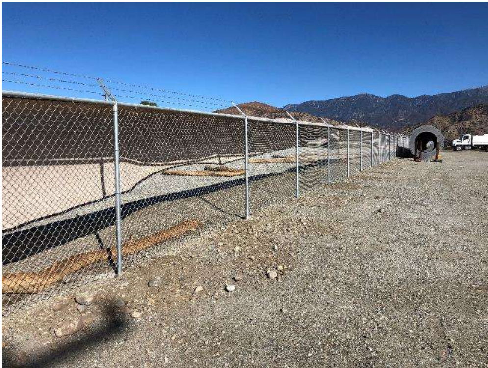
Photo 2 – Fiber rolls dislodged due to high winds at the Match MY (October 16, 2018).
