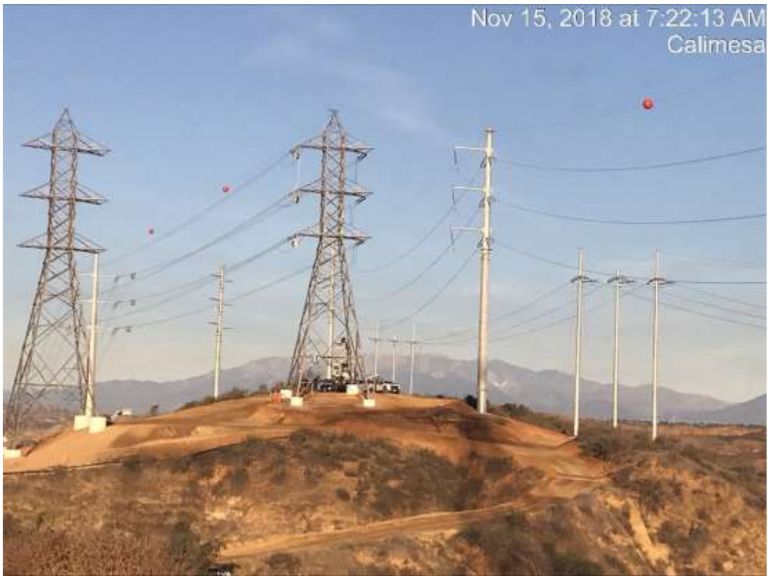
Photo 5 – Marker balls have been installed in the Segment 4 tower spans as recommended by the FAA. (November 15, 2018).
