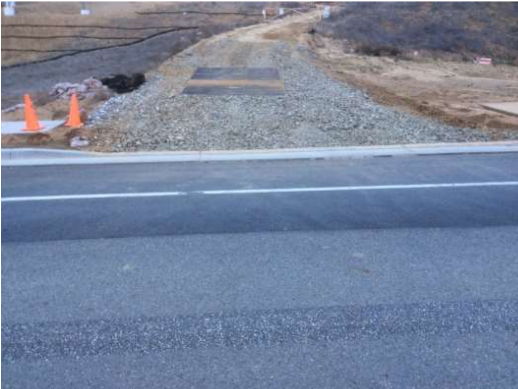
Photo 7 – Stabilized entrance after clean-up and maintenance at Palmer Ave, Segment 4. Photo courtesy of SCE.
