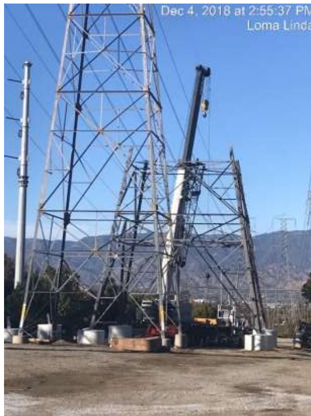
Photo 2 – New tower assembly and erection in Segment 1, part of the current outage (Move 1).
