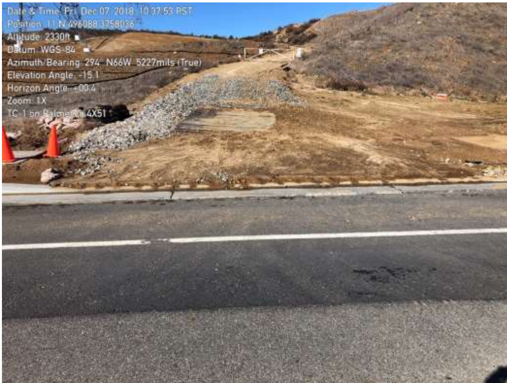
Photo 6 – After storm conditions of the stabilized entrance along Palmer Ave in Segment 4. Photo courtesy of SCE.
