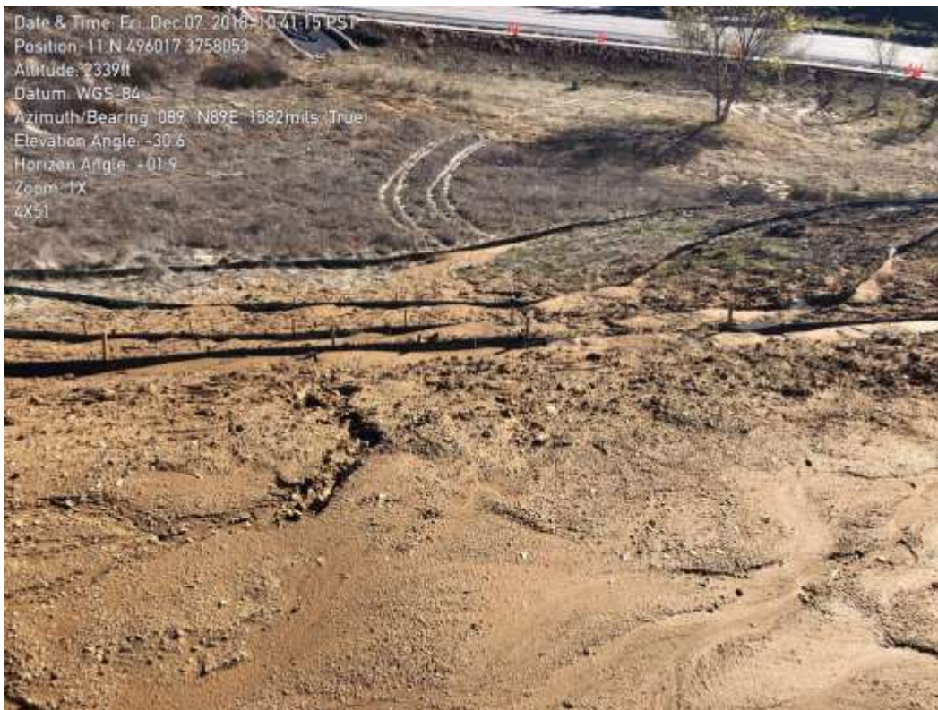
Photo 8 – Sediment build up on BMPs after storm at Segment 4 Site 4X51. Photo courtesy of SCE.
