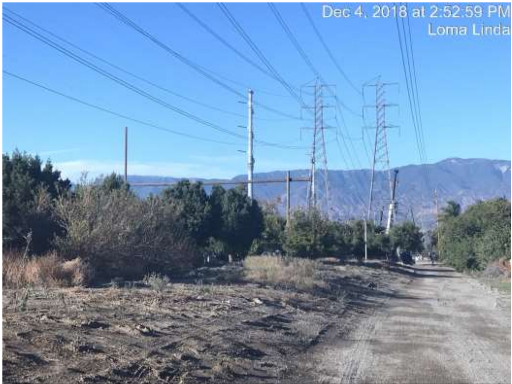
Photo 3 – Shoofly poles have been installed (steel monopole on left) to temporarily hold conductor during existing lattice tower wreck-out in Segment 1.
