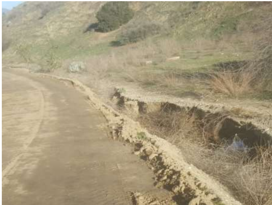
Photo 2 – Previously unidentified drainage near Site 3X55, Segment 3, reported to SCE by CPUC EM.
