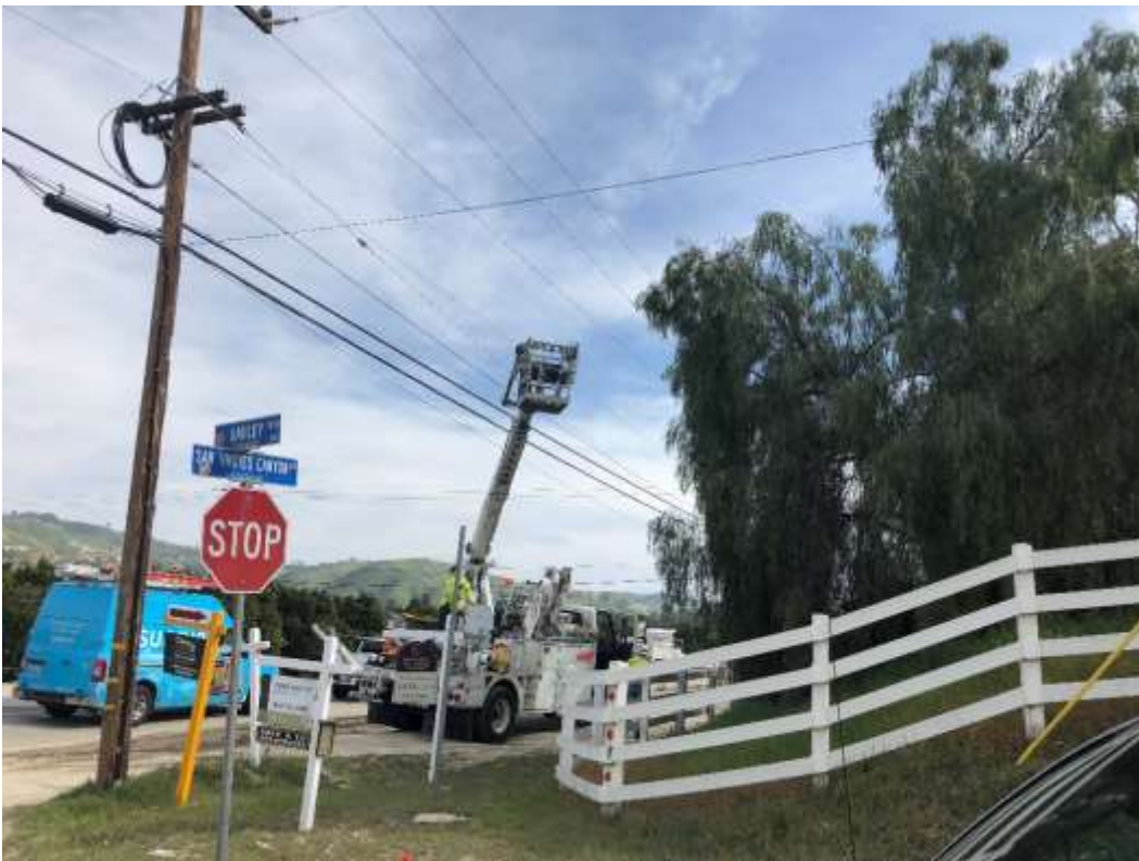
Photo 2 – SCE crew installing telecom fiber along San Timoteo Canyon Road for the El Casco Connection.
