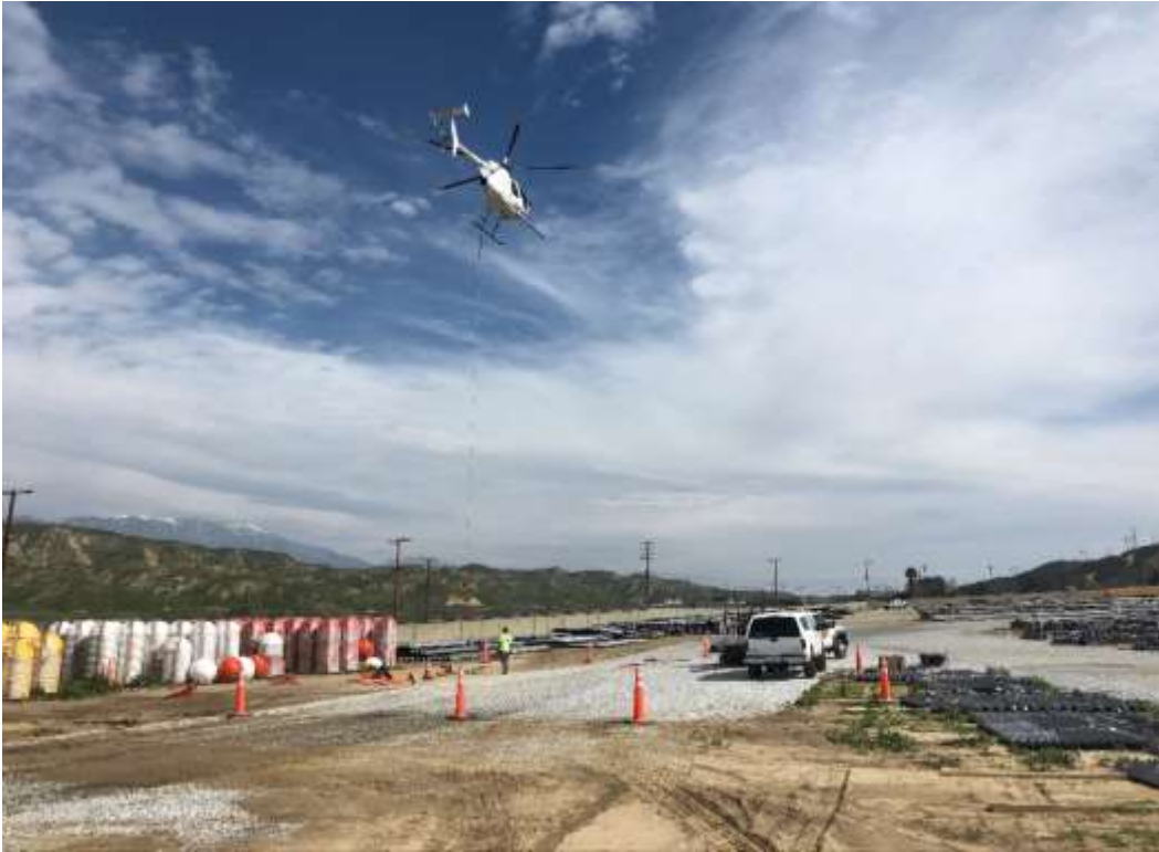
Photo 1 – Helicopter operations supporting wire installation and removal at the Poultry Yard on San Timoteo Canyon Road.
