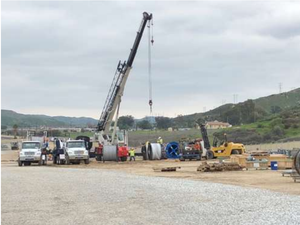
Photo 1 – Reels of conductor were delivered and unloaded at the Poultry Yard on San Timoteo Canyon Road.
