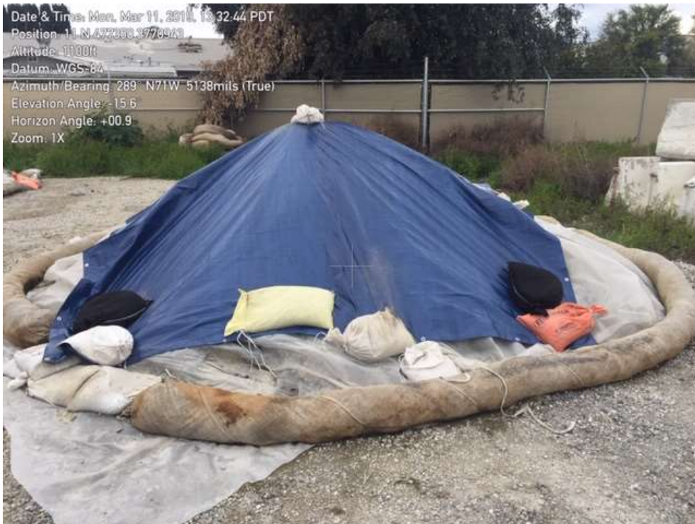
Photo 2 – Project Inspectors identified the need for stockpile cover replacement at the Mountain View Yard. The CPUC EM confirmed that the cover was replaced. Photo courtesy of SCE.
