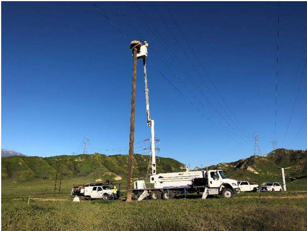
Photo 6 – Active red-tailed hawk nest relocated to installed nesting platform at Site 3X06-3X07 (March 13, 2019).
