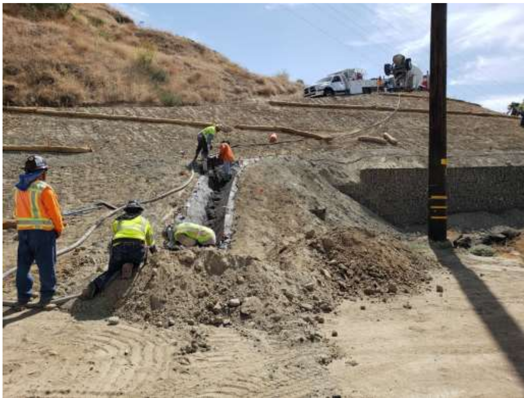
Photo 2 – Concrete pour for the v-ditch at Construction Area 2N32 on Segment 2 (September 9, 2019).
