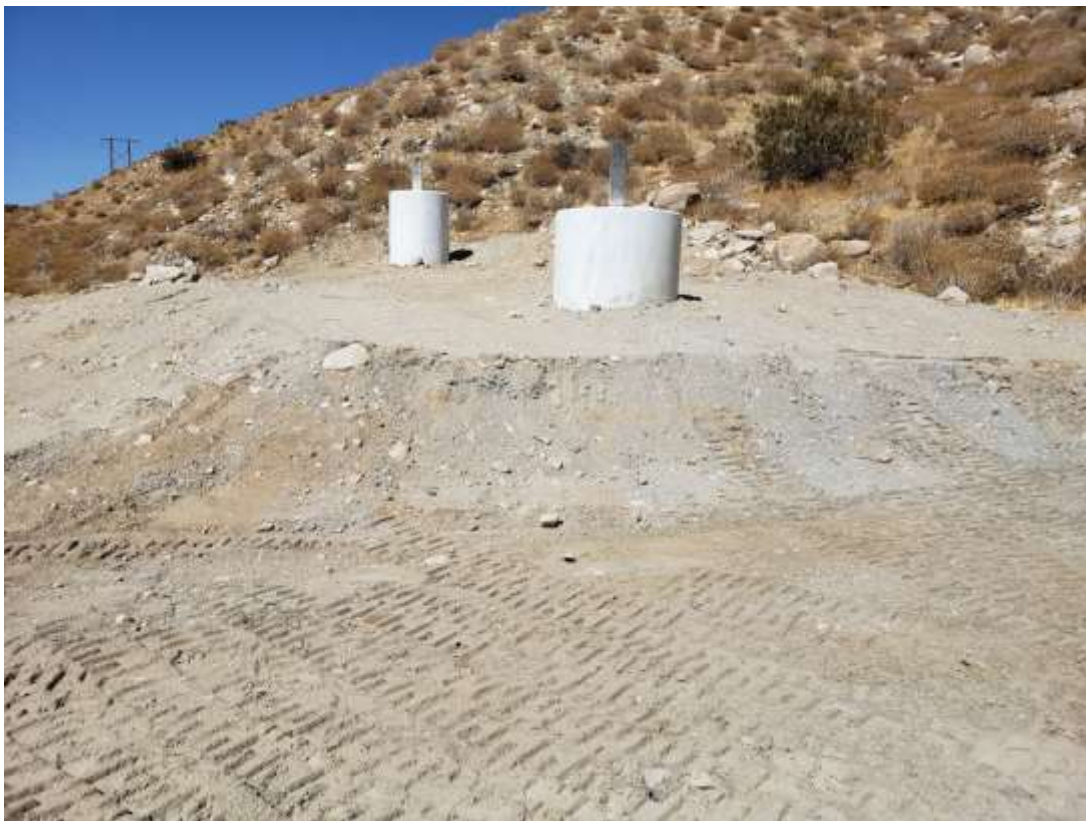
Photo 4 – Concrete slurry spreading level 1 incident on Segment 6 (September 24, 2019).
