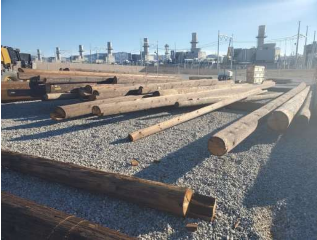
Photo 1 –Treated wood poles stored improperly at the Devers MY (October 21, 2019).
