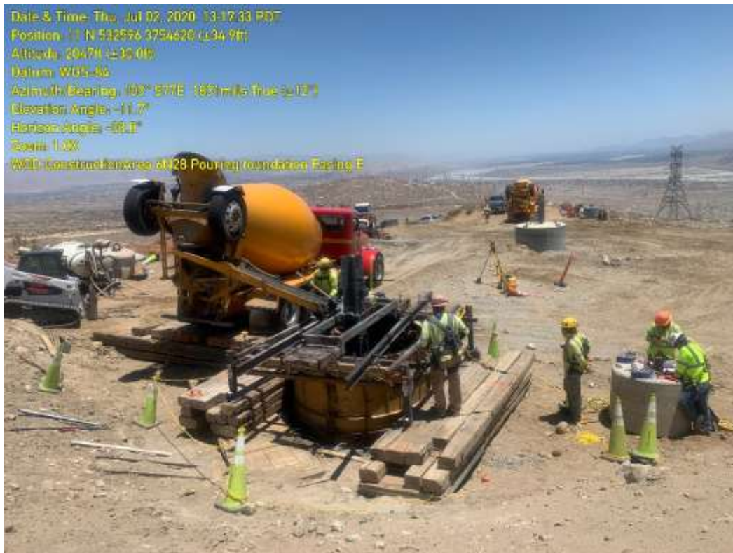
Photo 4 – Foundation activities at Construction Area 6N28, Segment 6 (July 2, 2020) (Photo courtesy of SCE).
