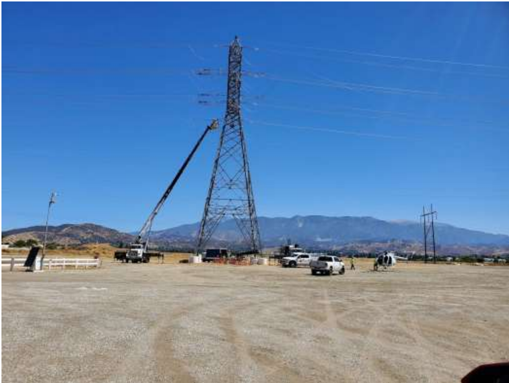
Photo 4 – Wire stringing activities and Helicopter Landing Zone at Construction Area 4X35, Segment 4 (July 15, 2020).
