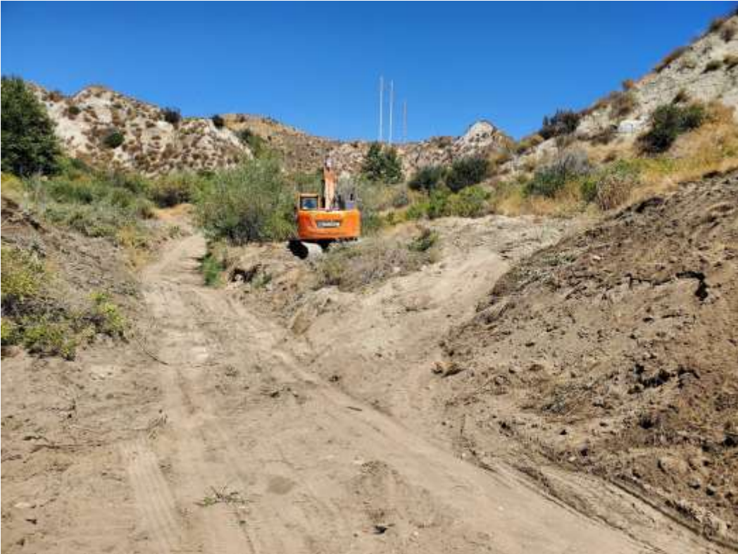
Photo 4 – Vegetation clearing at wet crossing on access road to Construction Area 4X04, Segment 4 (July 29, 2020).
