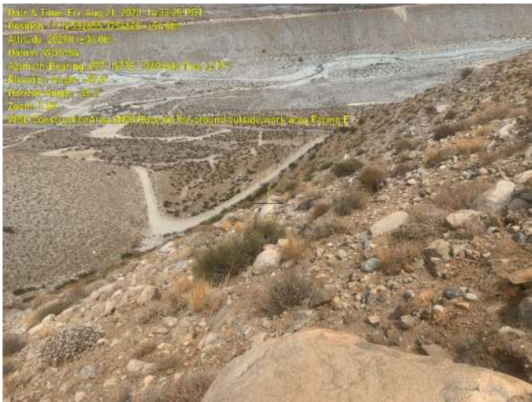
Photo 6 – OPGW rope drop near at Construction Area 6N28, Segment 6 (August 21, 2020) (Photo courtesy of SCE).
