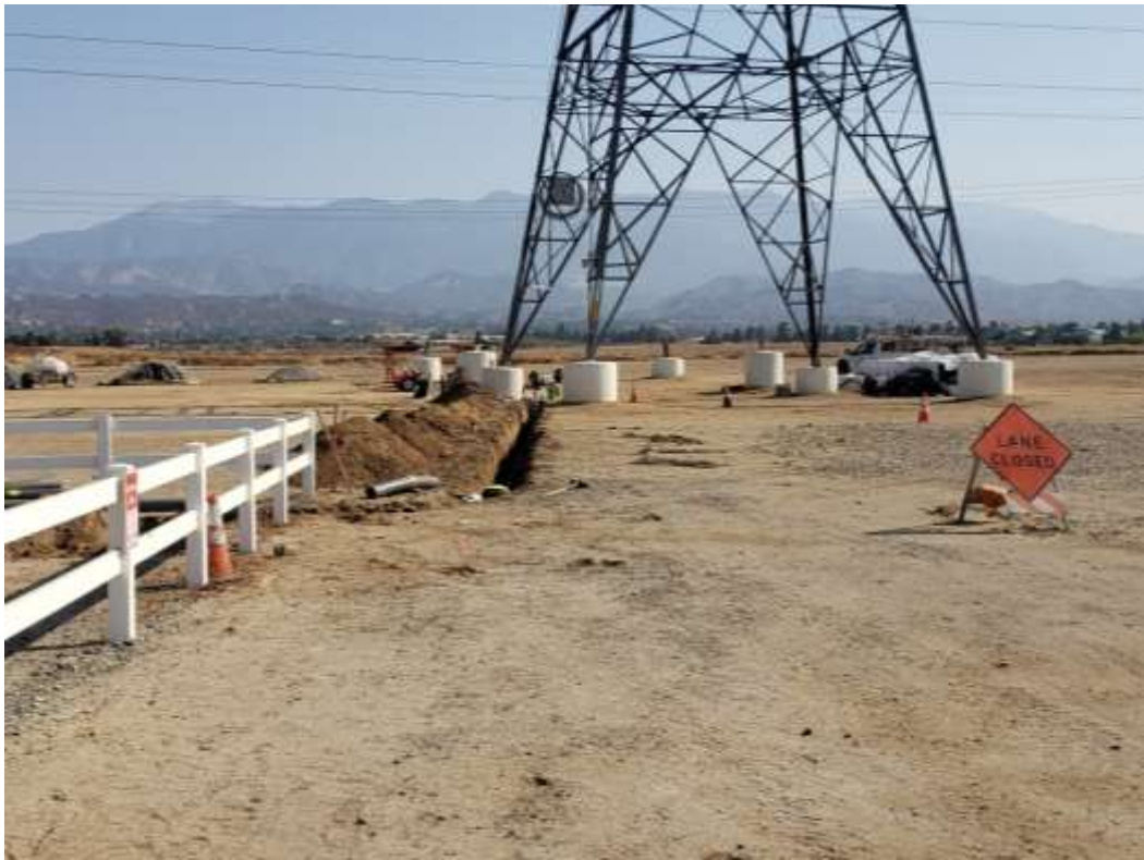
Photo 3 – Conduit installation activities at Construction Area 4X35, Segment 4 (August 21, 2020) (Photo courtesy of SCE).
