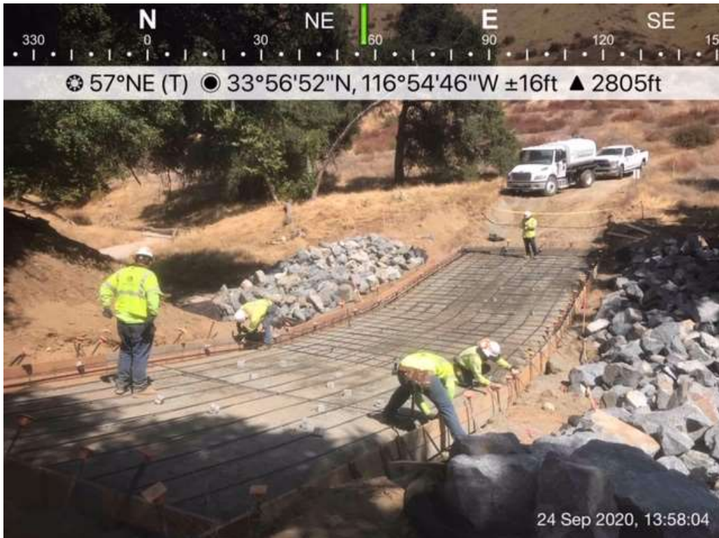
Photo 2 – Wet crossing installation on access road to Construction Area 4N12, Segment 4 (September 24, 2020) (Photo courtesy of SCE).
