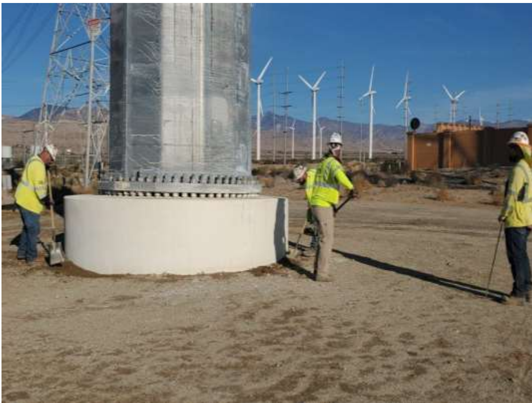
Photo 6 – Foundation compaction activities at Construction Area 6X08, Segment 6 (Photo courtesy of SCE) (October 8, 2020).
