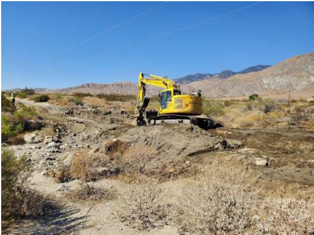
Photo 5 – Grading activities at wet crossing on access road to Construction Area 6N42, Segment 6 (October 13, 2020).
