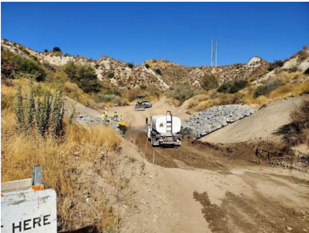
Photo 4 – Grading activities at wet crossing on access road to Construction Area 4X04, Segment 4 (October 12, 2020).
