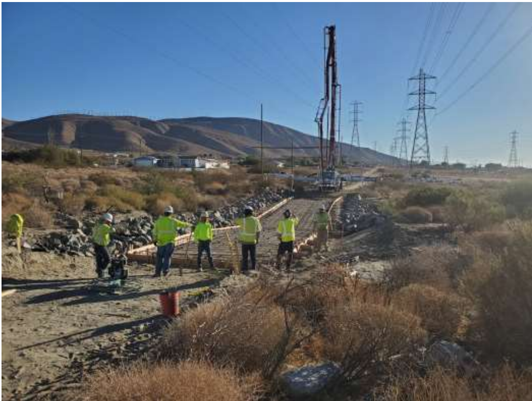
Photo 6 – Wet crossing installation on access road to Construction Area 6X42, Segment 6 (October 29, 2020).
