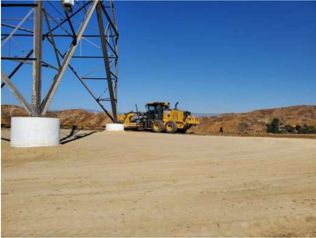
Photo 1 – Site restoration and berm punch-list activities at Construction Area 2N18, Segment 2 (October 28, 2020).
