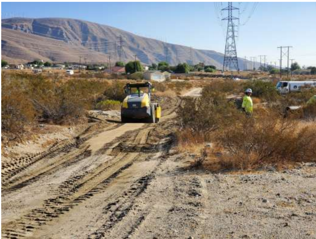
Photo 6 – Wet crossing grading on access road to Construction Area 6X41, Segment 6 (November 12, 2020).
